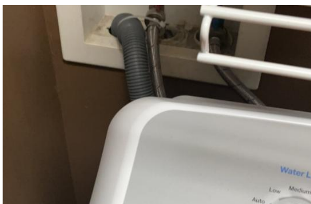
Photo 116: Water supply and drain
