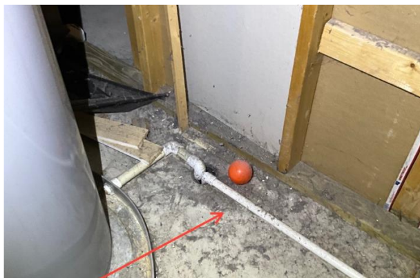
Photo 120: Dryer lint was observed on the floor behind the water heater and near the furnace
