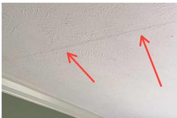
Photo 104: Normal settlement cracking in common area ceiling
