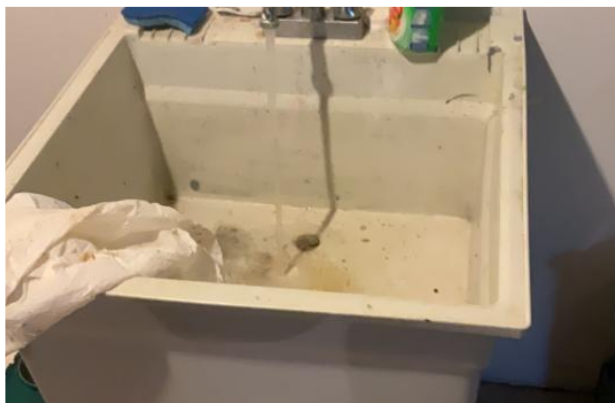
Photo 114: Functioning laundry sink
