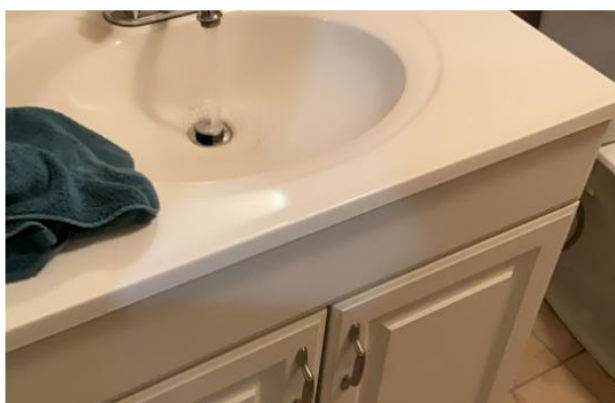
Photo 76: Functioning downstairs, bath-room sink and toilet
