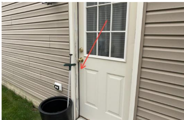
Photo 13: Peeling paint around man door
