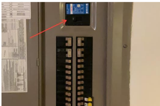
Photo 60: Main service disconnect
