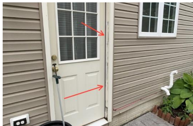
Photo 12: Peeling paint around mandoor
