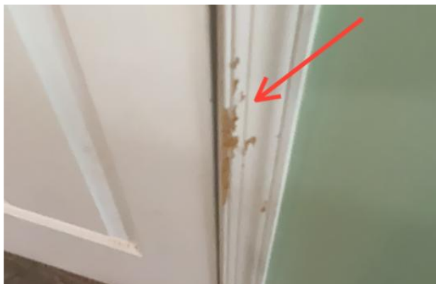
Photo 95: Damage to trim in livingroom
