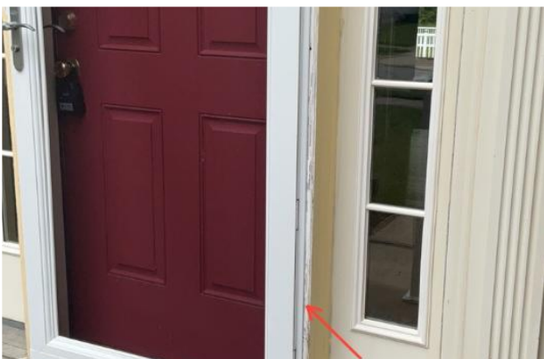
Photo 11: Peeling paint around front door
