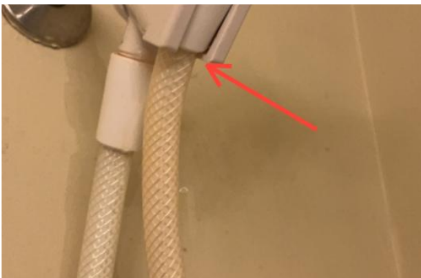
Photo 80: Shower head leaks in upstairs bathroom
