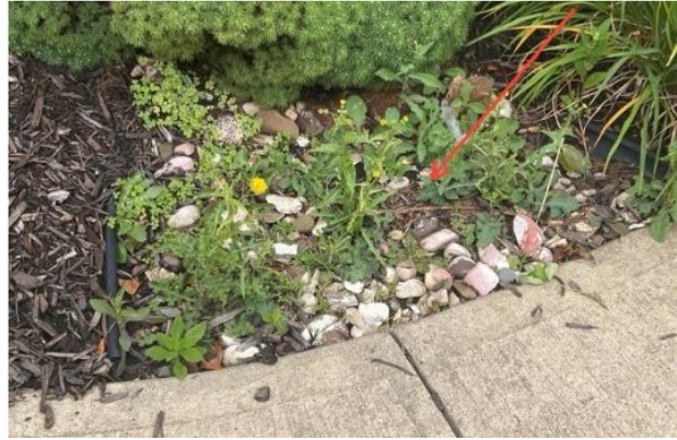
Photo 16: Front downspout drains into flower bed
