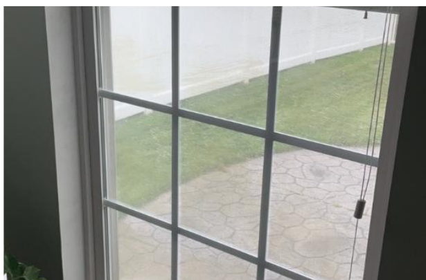
Photo 105: Loss of thermal seal in dining room
