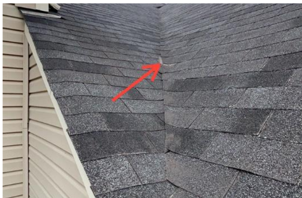
Photo 24: Front roof damaged shingle
