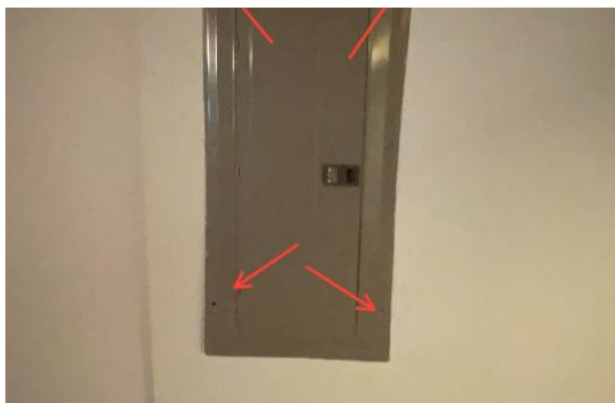
Photo 59: Panel was missing four screws
