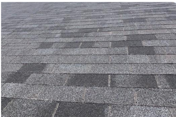
Photo 25: Lifted shingle front roof
