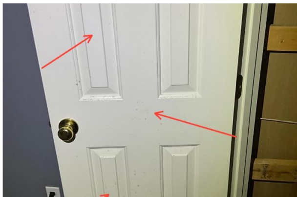
Photo 88: Signs of previous moisture were present on the inside of the door leading to the main water shut off. The stains were dry at the inspection.
