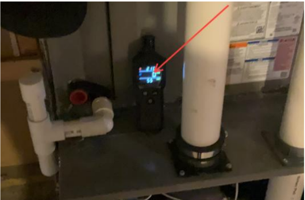
Photo 125: No CO gases were detected at inspection
