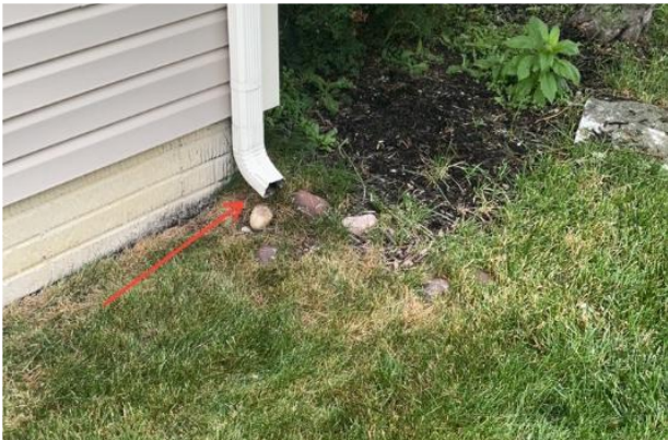
Photo 20: Left front corner of home downspout draining at foundation
