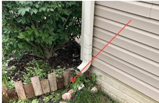
Photo 21: Right front corner of garage draining at foundation
