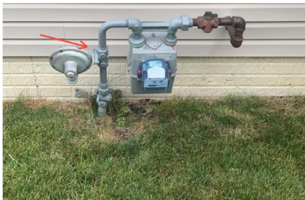
Photo 14: Gas meter is tilted and out of level
