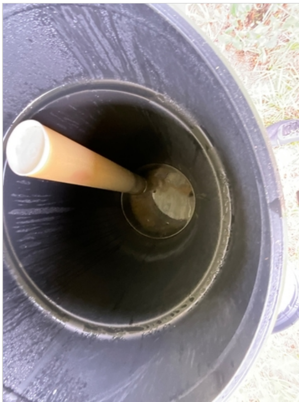
Empty salt tank
