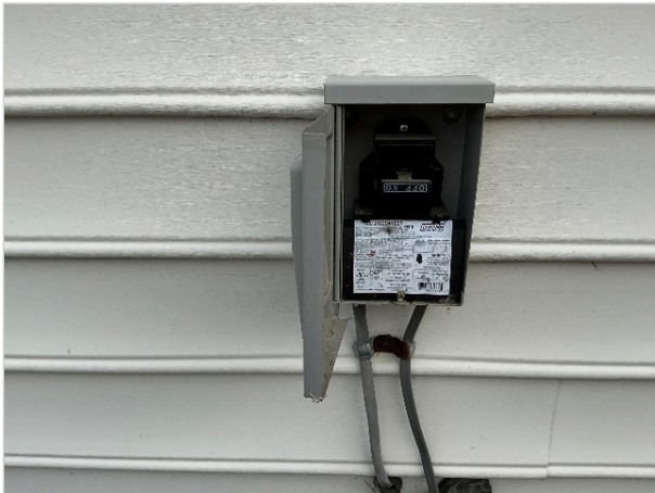
AC shut off switch
