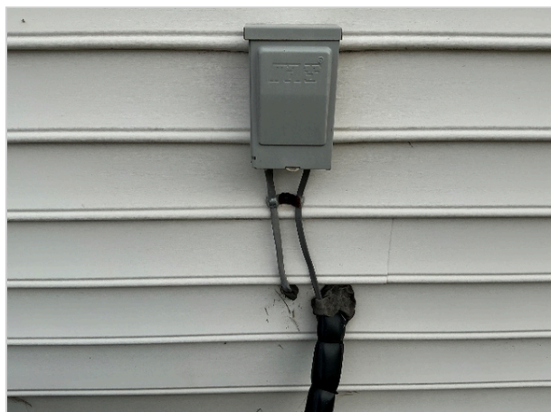
AC shut off box
