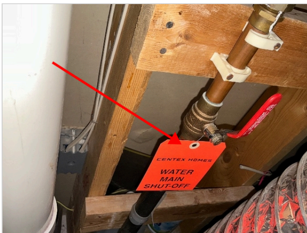
Water Main Shut off
