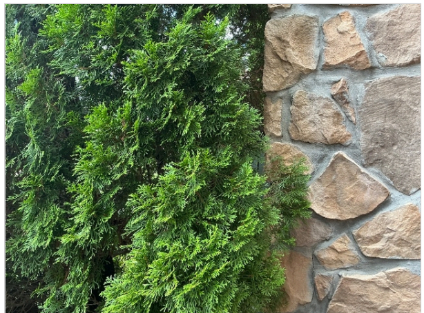
Overgrowth of Shrubs near adjacent unit
