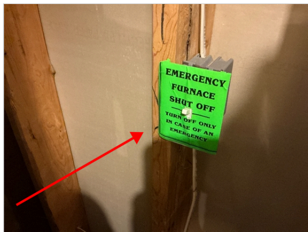
Furnace Shut off
