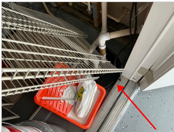
Sump Pump in Utility Closet in Garage
