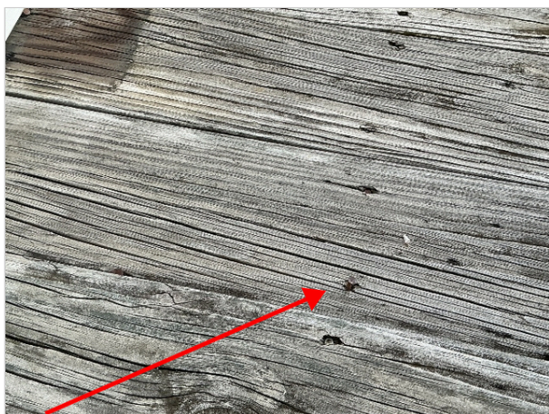
Loose nailing on Deck Surface
