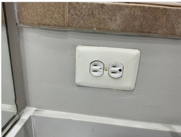
Bathroom Electric Receptacle
