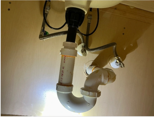
Beneath the sink of third floor hallway bathroom
