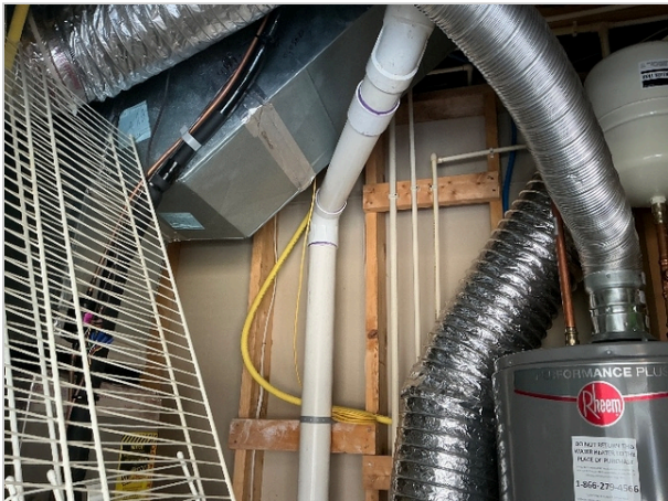
Water Heater Exhaust Duct
