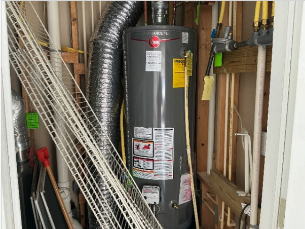
Water Heater in Utility Closet
