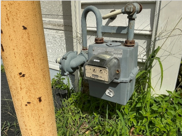
Gas Meter on left side of home
