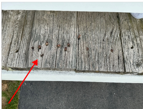
Nails near Deck Edge
