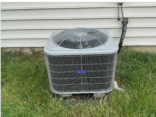
Outside condensing unit
