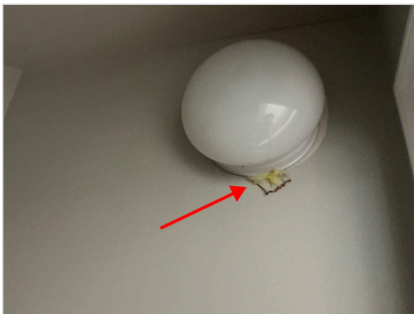
Light in storage closet in basement under staircase
