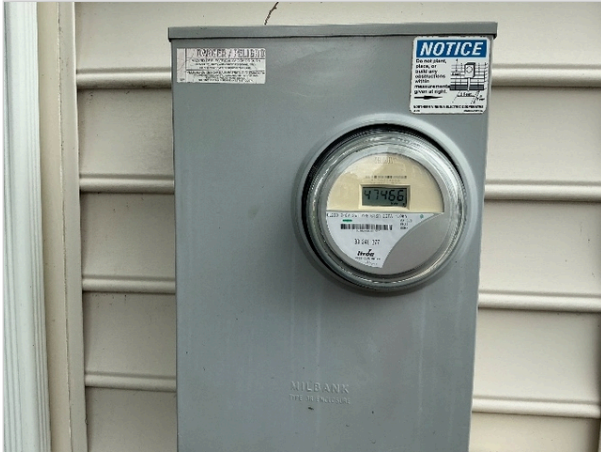
Electric Meter on Left side of Home
