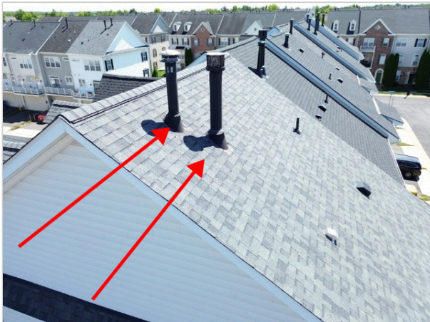
Gas Burning B Vents
