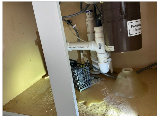
Leak below kitchen sink
