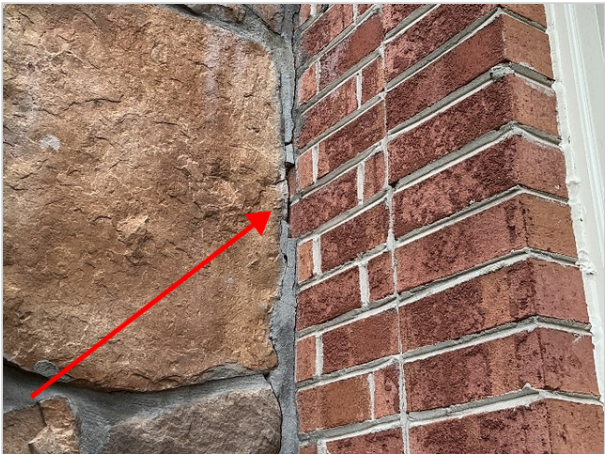
Cracking of Mortar where adjacent unit meets brick cladding
