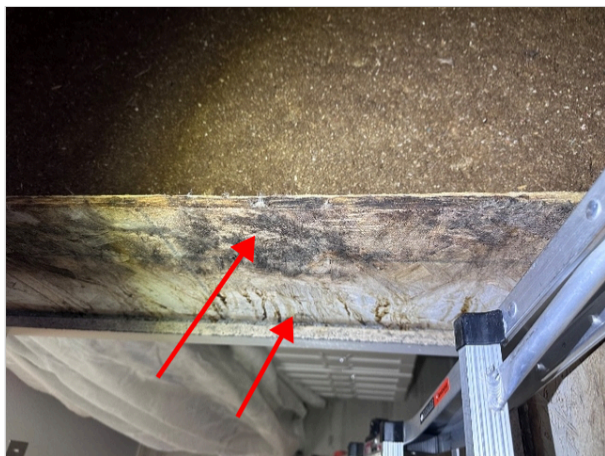
Black Substance and evidence of dripping
