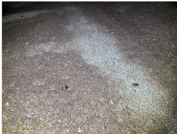
Humidity affected insulation
