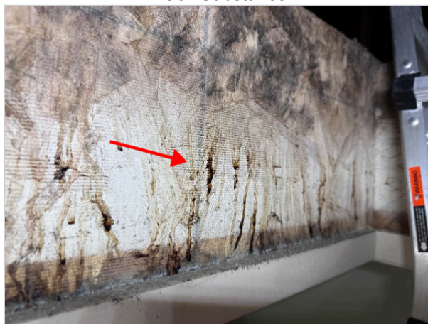
Drips in attic scuttle are evidence of moisture
