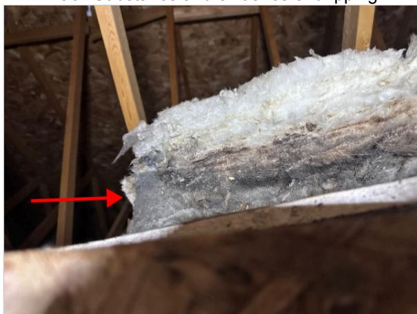
Black Substance in Attic Scuttle Insulation
