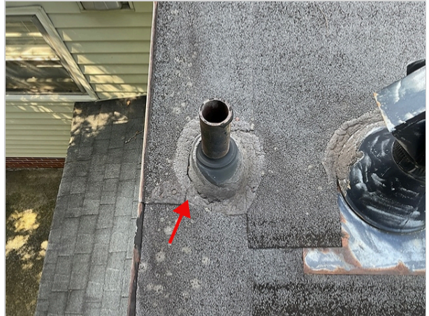
Cracked sealant on plumbing boot in rear addition
