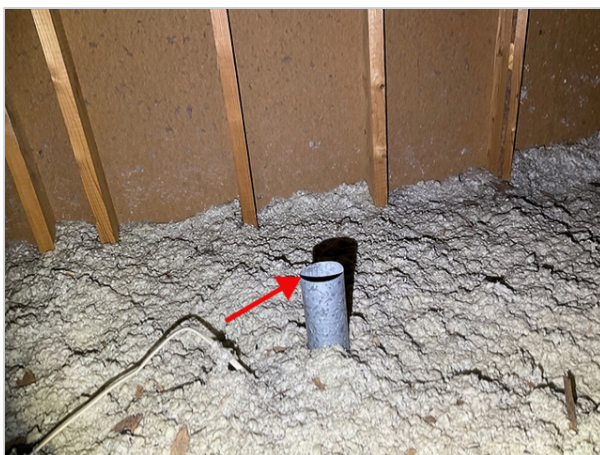
Bathroom bath fan vents into attic
