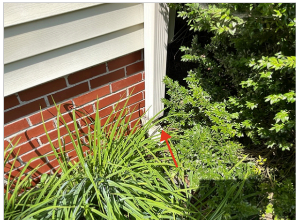
Downspout drains too close to foundation
