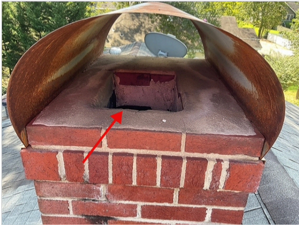
Open chimney. Cover to prevent animal intrusion
