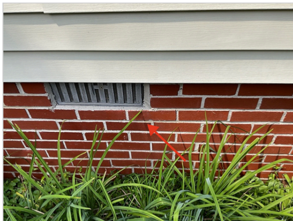
Small crack in foundation on rear of structure
