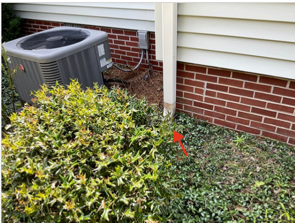
Downspout drains too close to foundation
