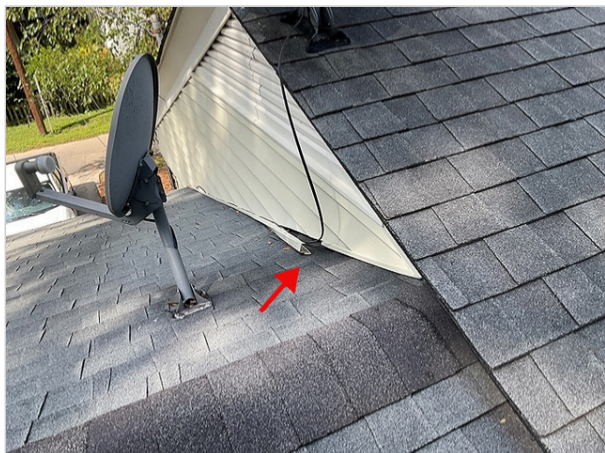
Loose siding over carport transitions
