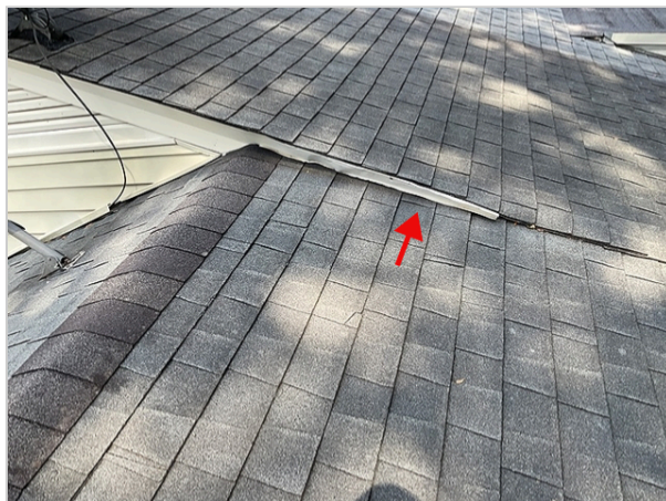
Loose siding over carport transitions
