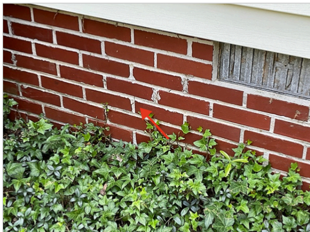
Small crack in foundation on left side of structure
