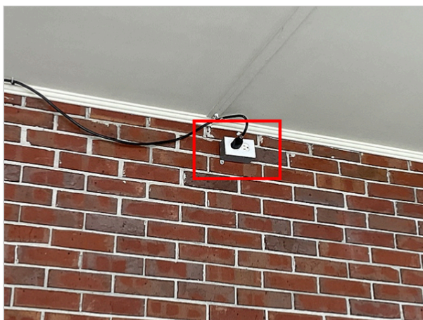
No cover on exterior outlet under carport
