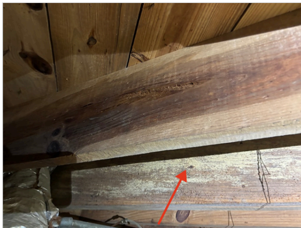
Mold like growth in crawl space
