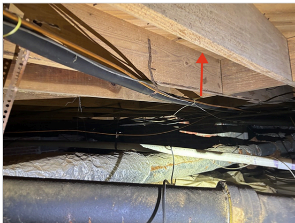
No insulation on subfloor in crawl space
