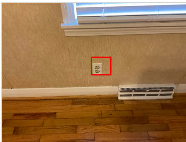
Two prong outlets in structure
