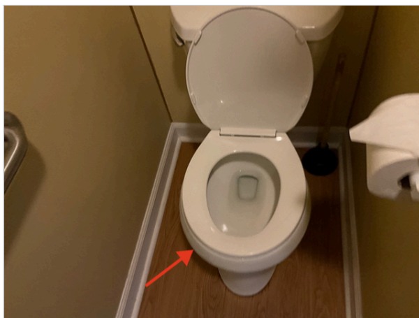
Loose toilet in primary bathroom
