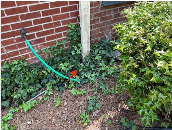
Downspout drains too close to foundation on front of structure
