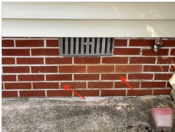
Small crack in foundation on rear of str
