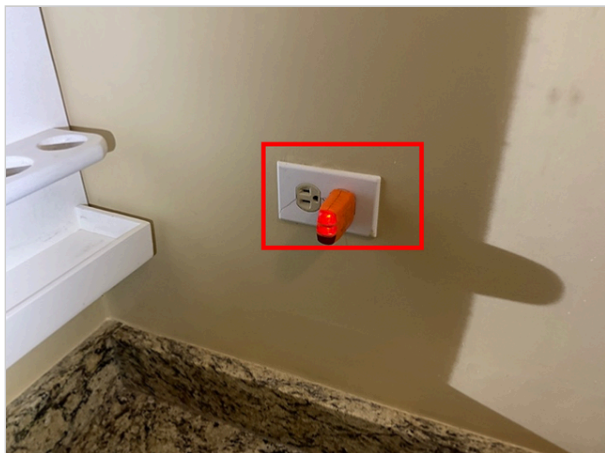
No GFCI protection in bathroom
