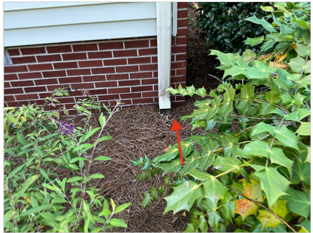
Downspout drains too close to foundation
