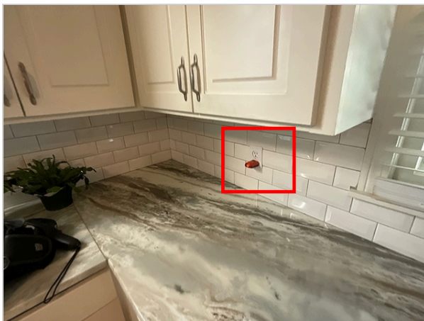
Kitchen lacks GFCI protection
