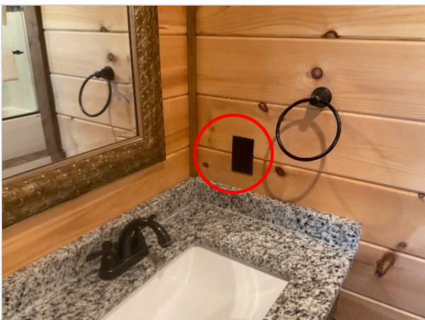
Left side master GFCI
