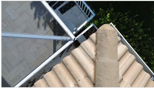
The gutters were in need of sealing at the corners.
