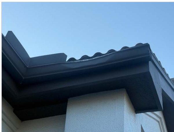
There was a damaged rain guard at the right of the home, in need of repair.
