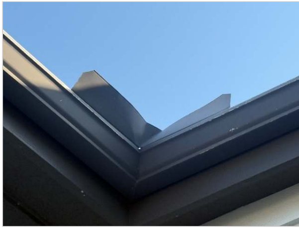
The gutter downspout extension was not attached and in need of repair.
