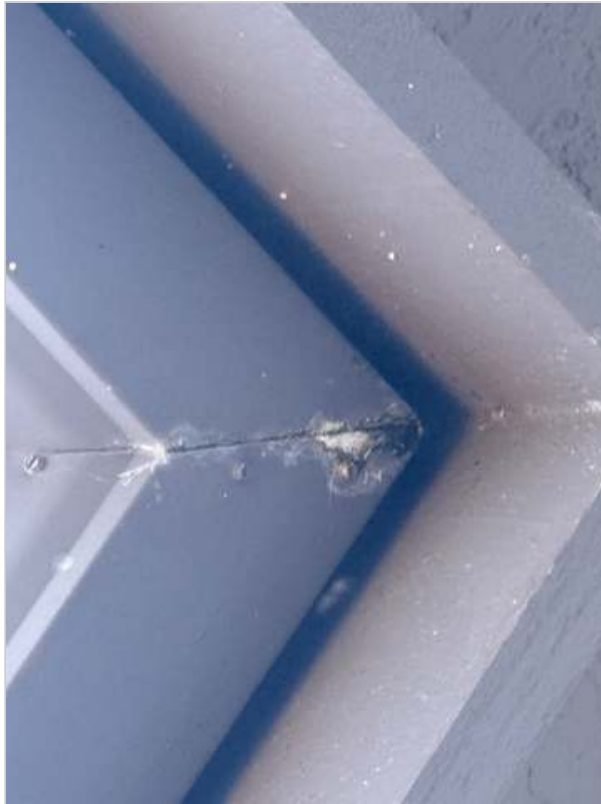
At the front left of the home, the gutter was damaged and in need of repair or replacement.
