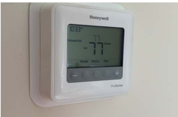
Photo 230: Second floor Honeywell
