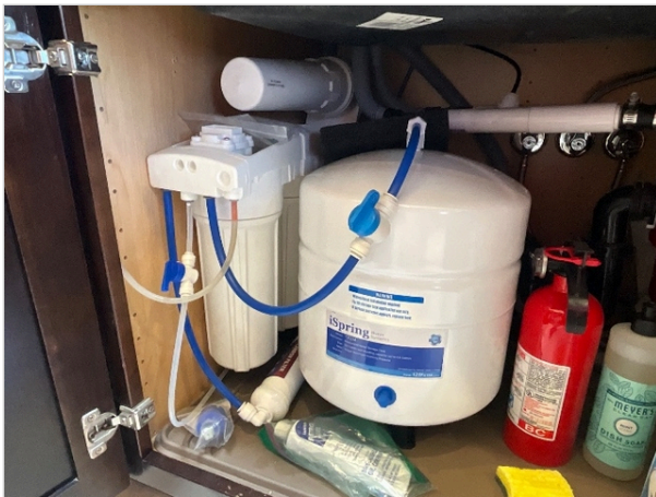
Water filtration system installed under kitchen sink
