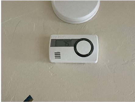
Carbon monoxide detector. In primary bedroom, eat end hallway.
