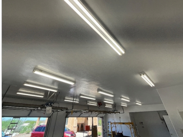
All garage ceiling lights with exposed bulbs
