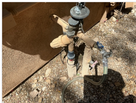
Back flow and shut off and control valve
