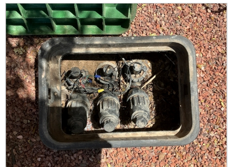
Control valve s
