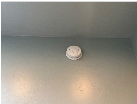
Smoke detector 1. In west end hallway,
