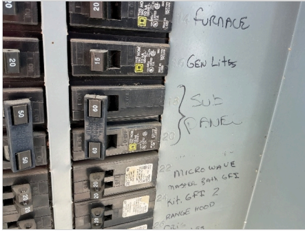
Sub panel disconnect
