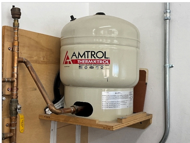
Water heater expansion tank
