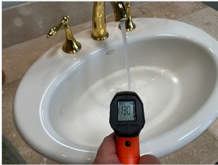
Measured water temperature
