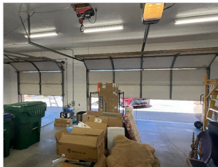
Properly balanced springs
