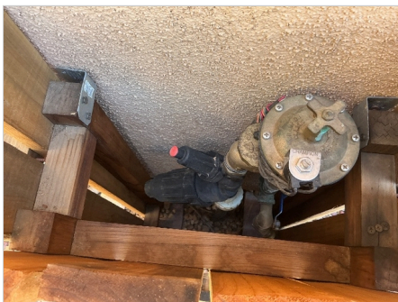
Back flow and shut off
