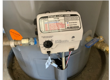
Water temperature monitors and setting
