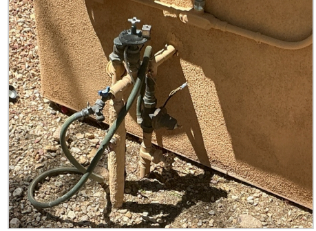
Access point and shut off and pressure regulator
