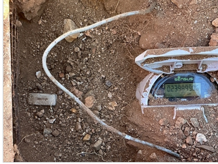
Meter and shut off
