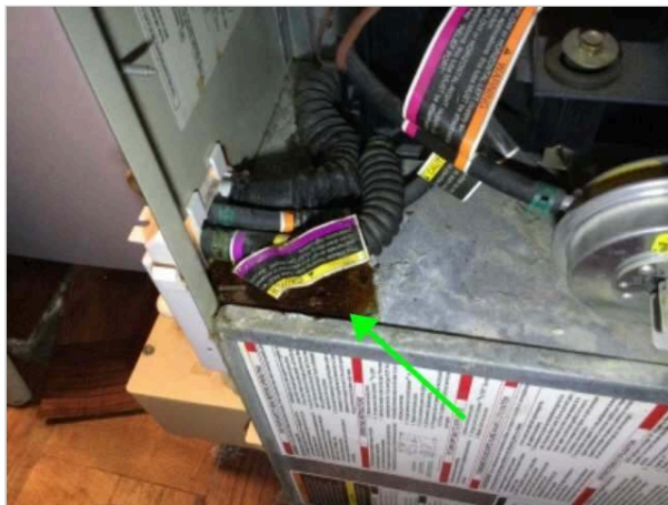
Water inside furnace
