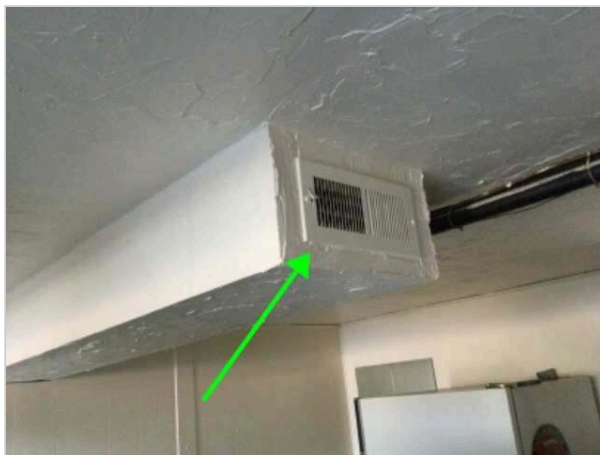
Open air vent in garage
