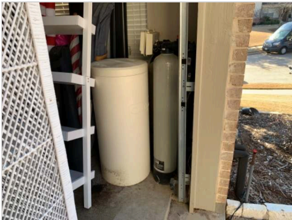
Water treatment system in garage
