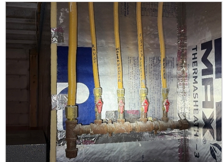
Gas lines in the basement
