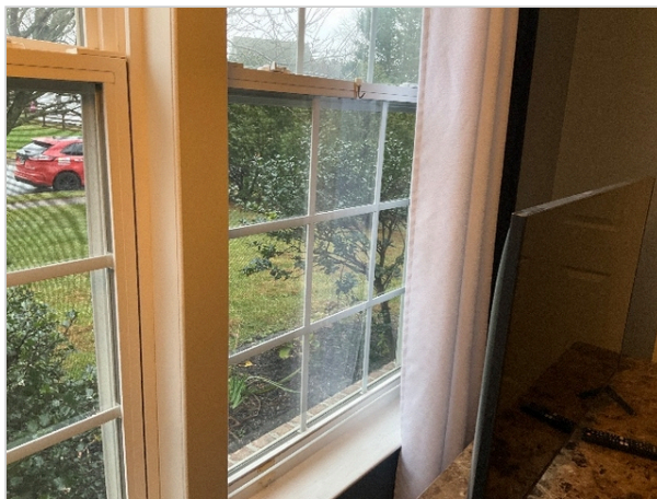
Once halfway shut, slams closed. Bedroom facing street.
