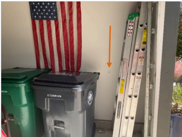
Dent in drywall
