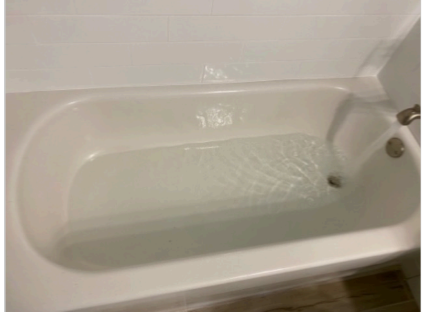
Hall bathroom drains slowly.
