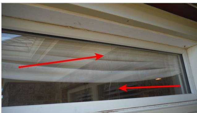
Cracked window pane-rear entry door
