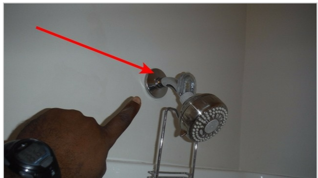
Upstairs bathroom shower stem
