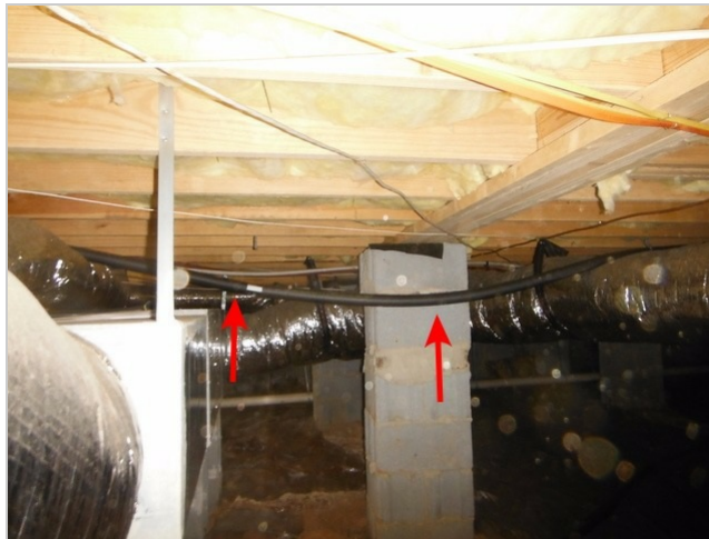
Water line not fully supported
