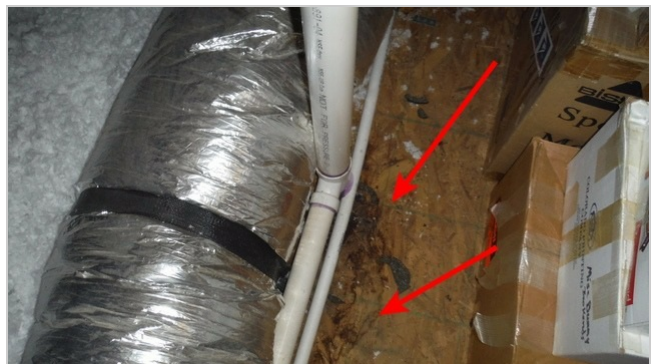
Deck staining below exhaust vent-attic
