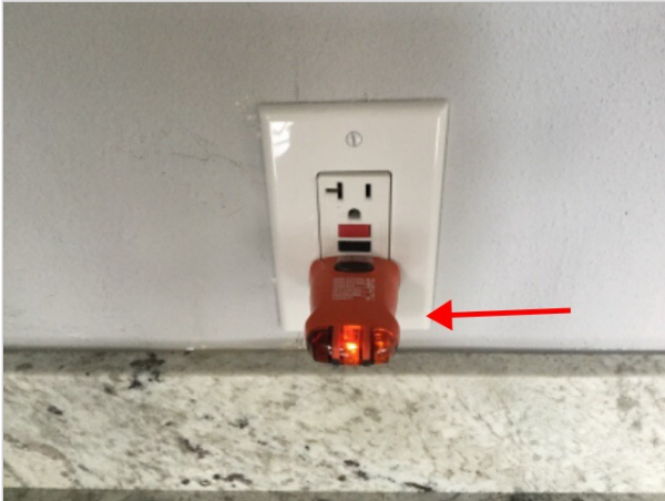
Kitchen GFCI by range
