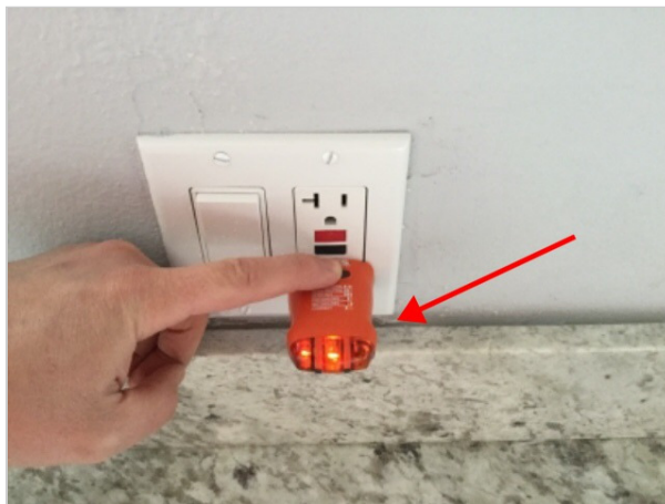
Kitchen sink GFCI
