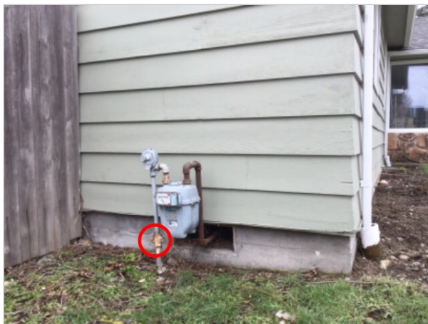
Main gas shut off valve
