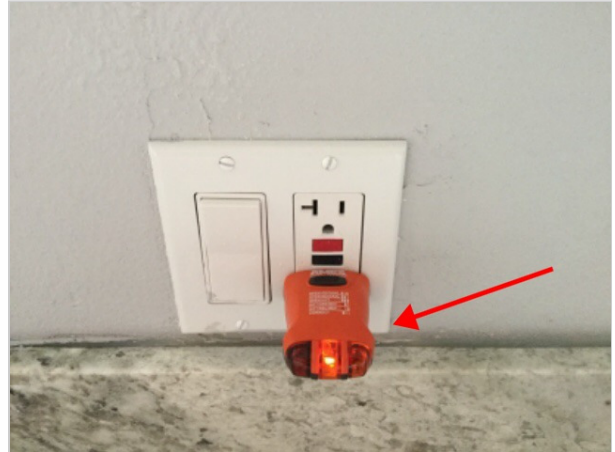
Kitchen GFCI by sink
