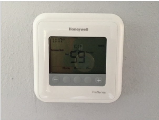
Thermostat settings at beginning of inspection
