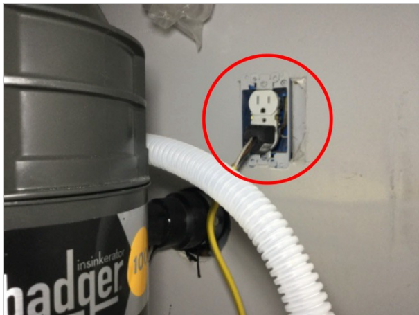
Dishwasher disposal outlet under kitchen sink
