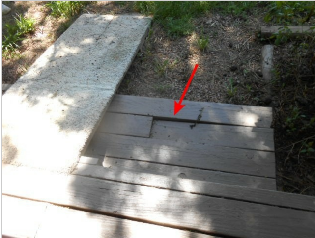
Loose or deteriorated deck board on the rear deck.
