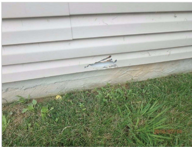
example of damaged siding
