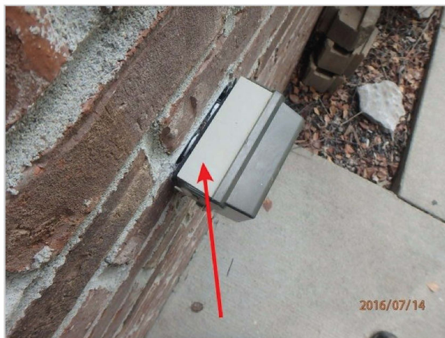
outlet is not properly covered
