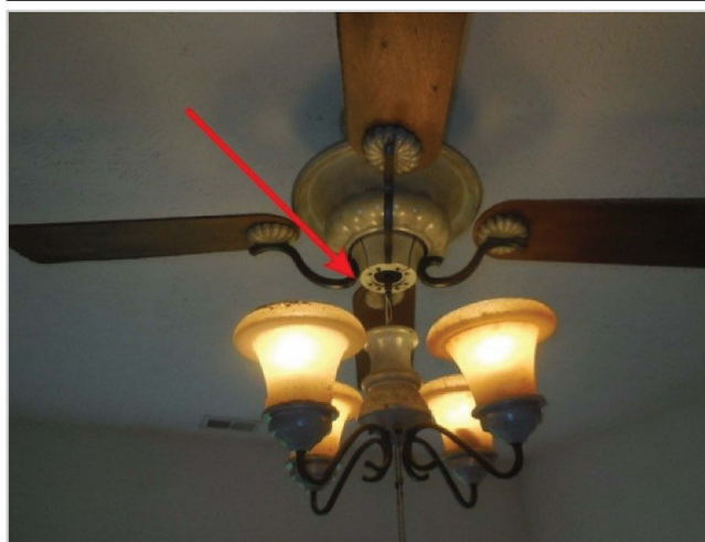
Loose light fixture.
