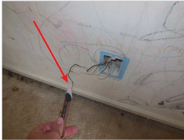
Exposed live wires.
