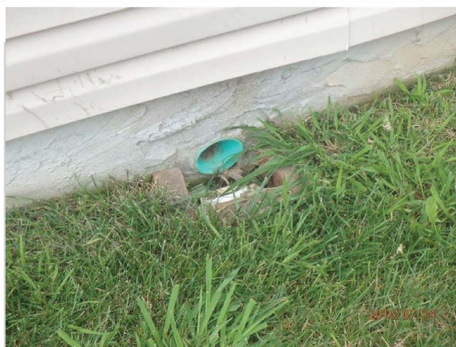
missing dryer vent cover
