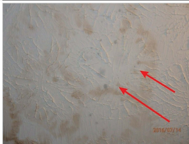
mold like growth in the garage
