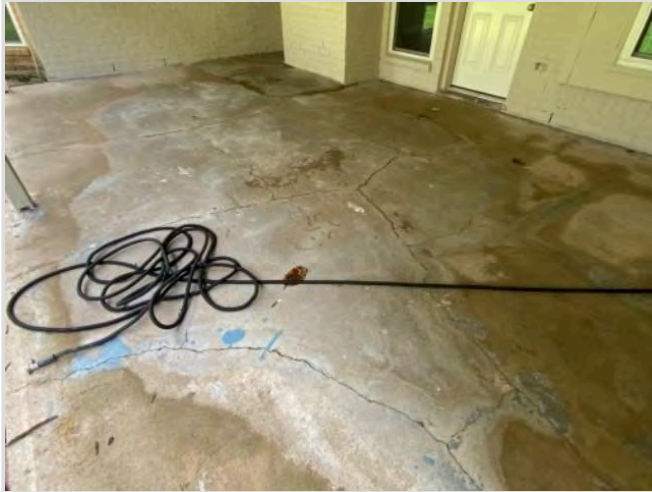
Cracks at non-structural rear patio floor
