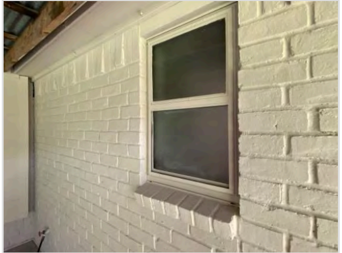
Missing screen (back porch)
