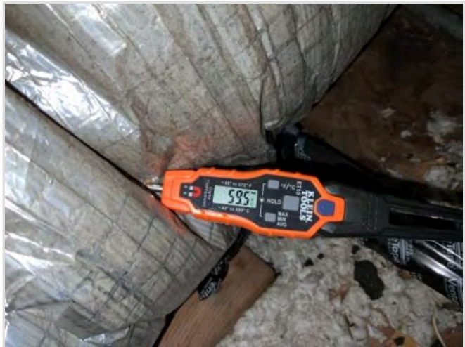
Supply air temperature 59.5 degrees
