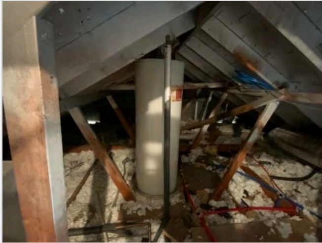
Water heater in attic
