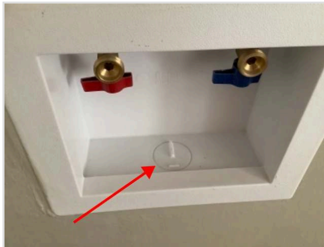
Laundry drain was not accessible
