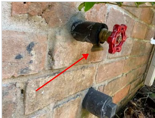
No back-flow prevention (left side)
