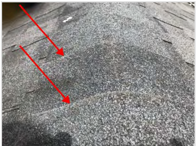
Exposed fiberglass at ridge shingles indicates significant wear
