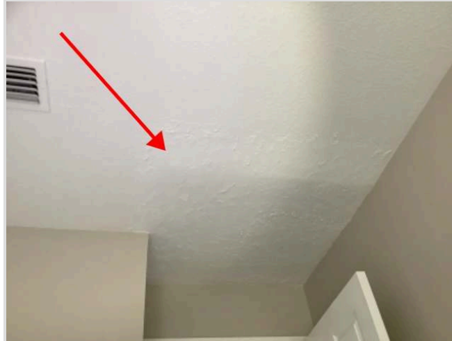
Previous ceiling repair (second floor front left bedroom)
