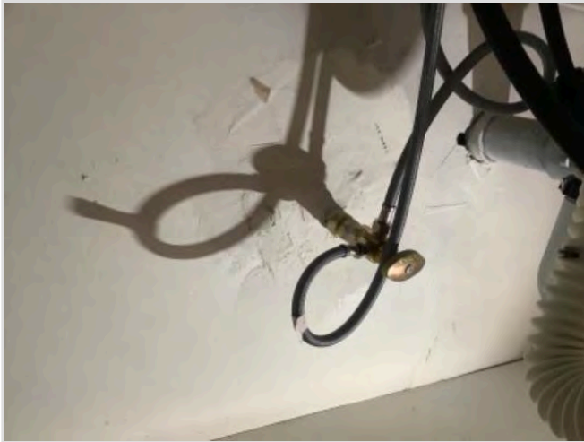
No hot water line (bar sink)
