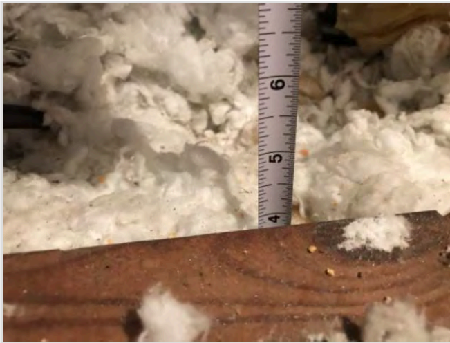
Average attic insulation depth was 4 inches or less
