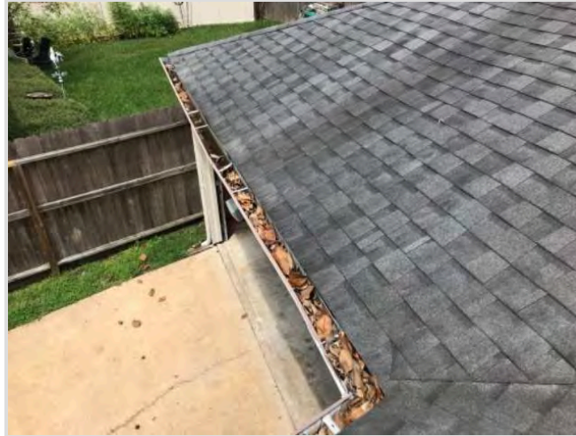
Debris in gutters (garage)
