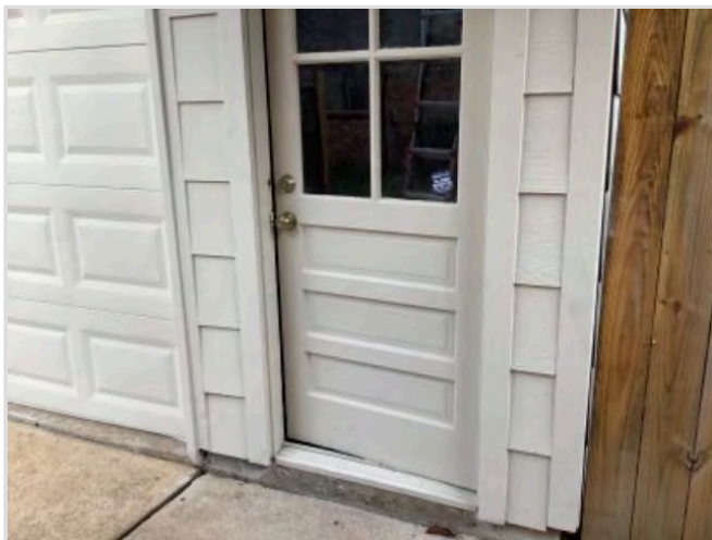
Would not latch in the closed position (garage access door)
