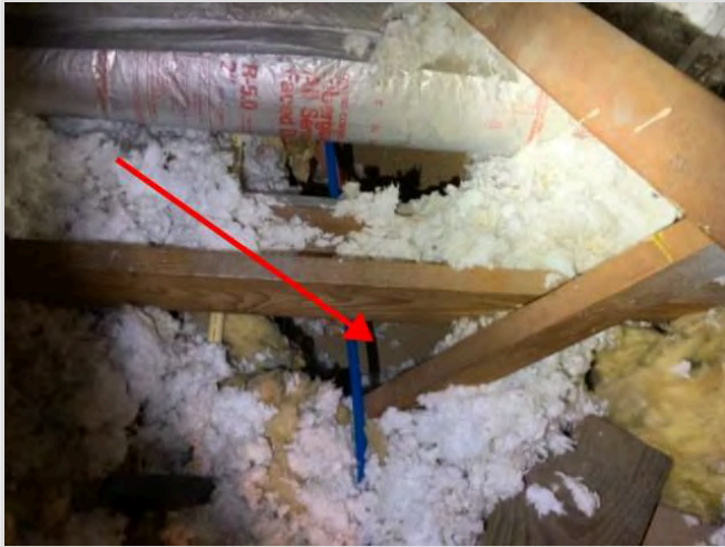
Missing insulation at dropped ceiling (behind water heater)
