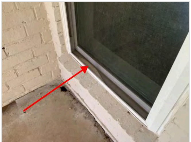
Damaged screen (back porch)
