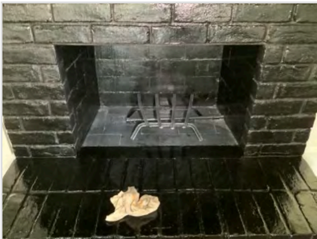
No screen installed at firebox opening
