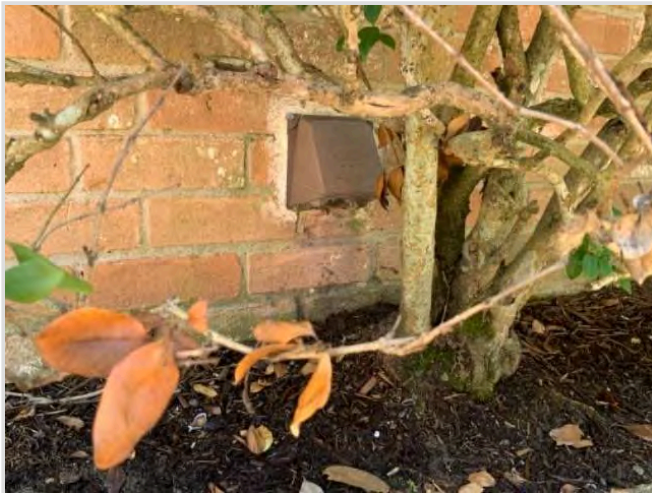
Dryer exhaust vent (left side)
