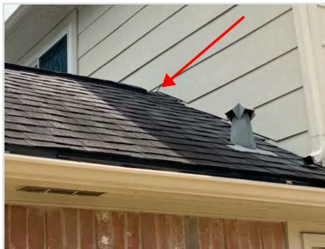
Joint or crack in siding is in need of routine caulk maintenance (rear)
