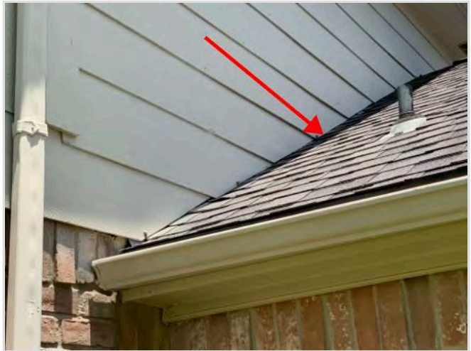
Siding in contact with roof covering (right side)
