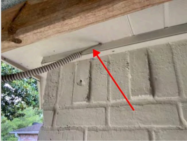
Wire outside of conduit (back porch)
