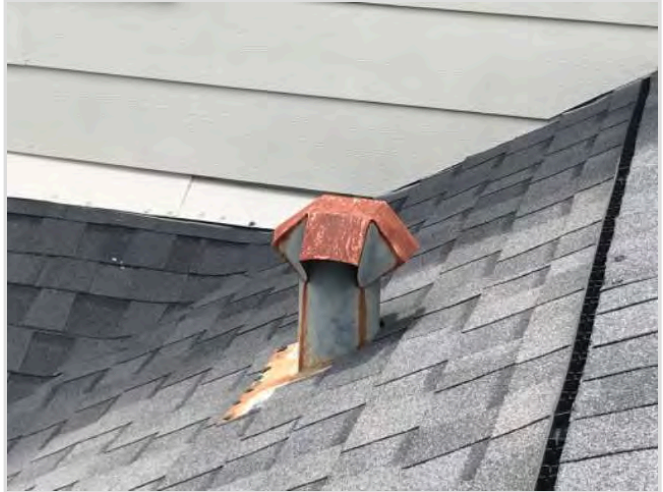
Rusted vent cover
