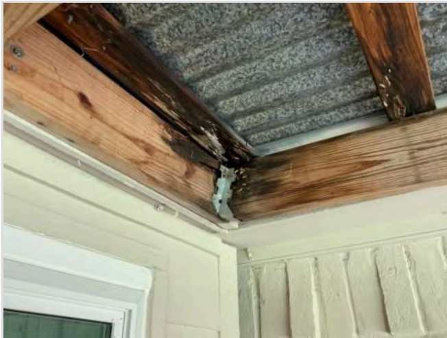
Signs of water penetration and wood rot (back porch joists)
