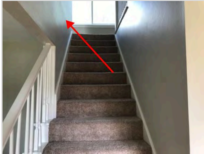
There was no continuous handrail at the upper portion of the stairs
