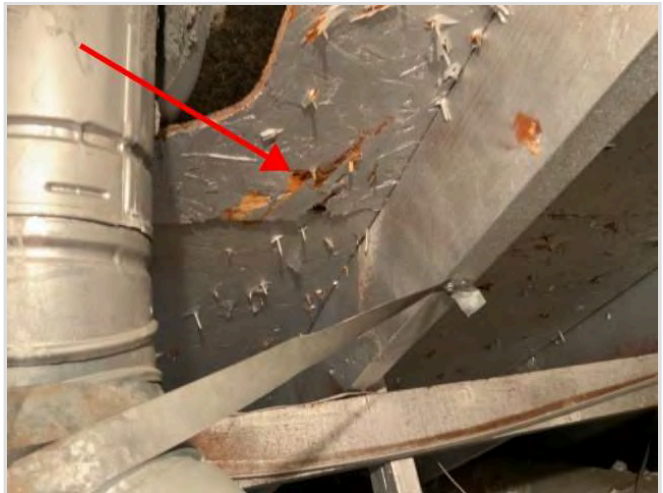
Damaged roof decking
