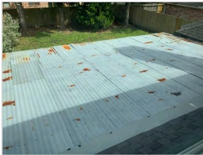
Rust on metal patio roof
