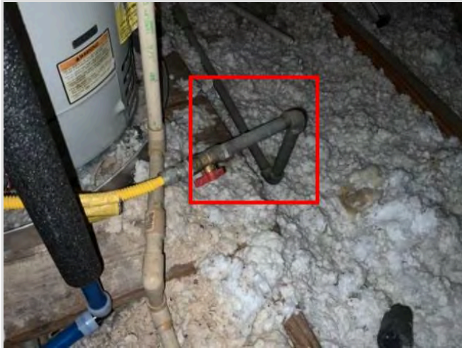
No sediment trap at water heater
