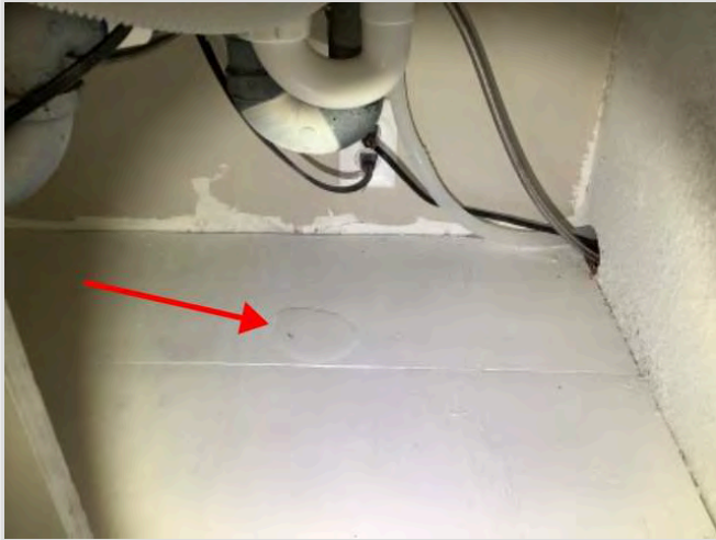
Leak (kitchen sink)
