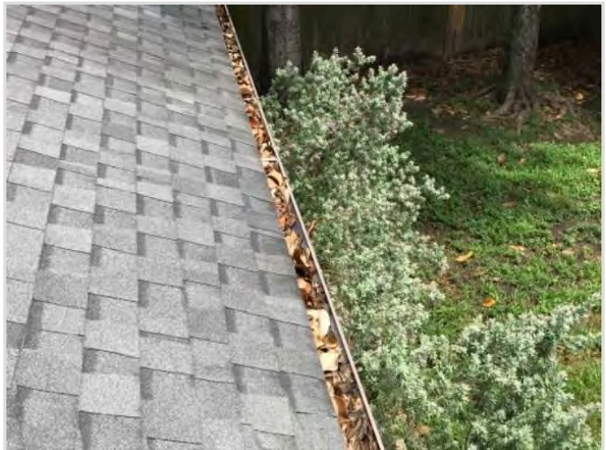
Debris in gutters (garage)
