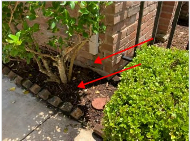
Missing the bottom elbow piece and splash pad (left side)
