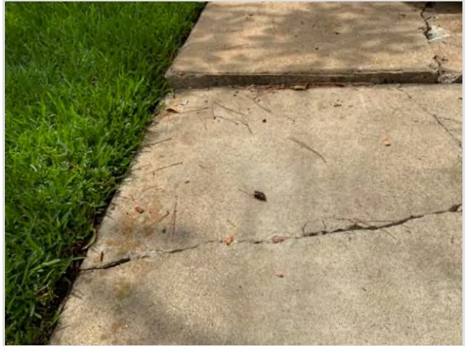
Cracks in driveway
