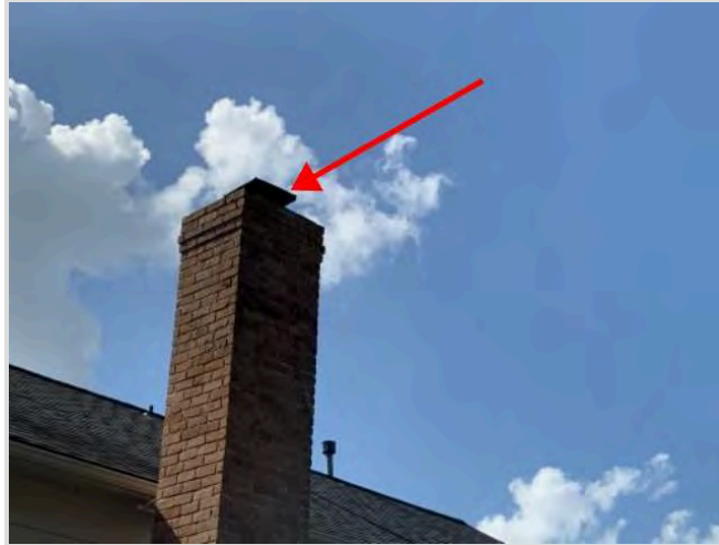
Rust at chimney cap and spark arrestor
