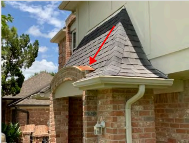
Rusted metal roof (above front porch)
