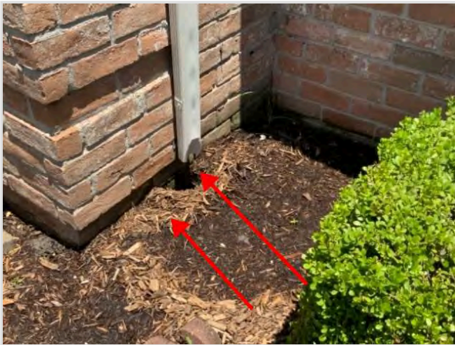
Missing the bottom elbow piece and splash pad (front)
