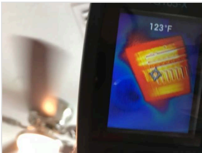
Appropriate temperature reading during heat cycle (second floor front right bedroom)
