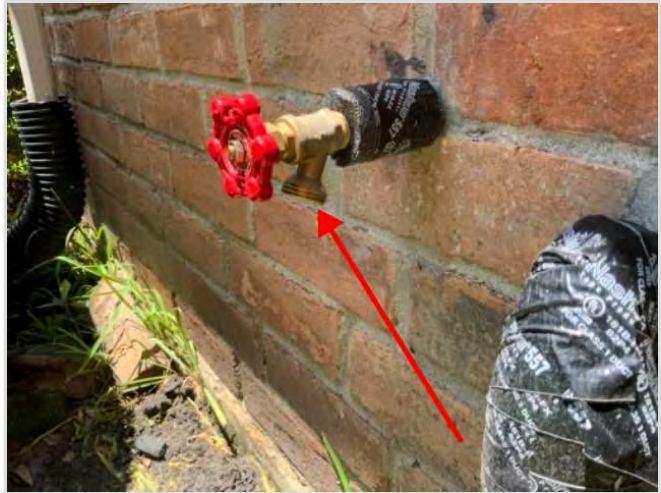
No back-flow prevention (right side)
