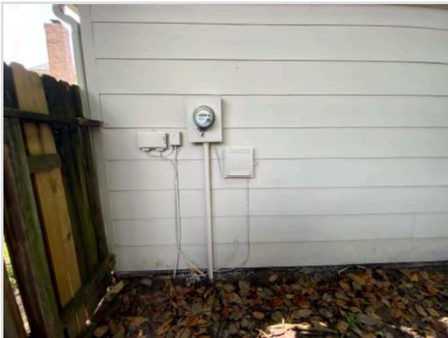
Electric meter (back of garage)
