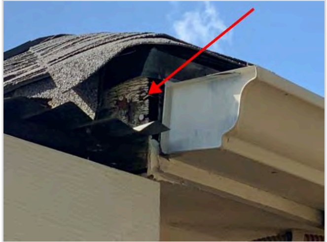
Wood rot at fascia above metal back patio roof
