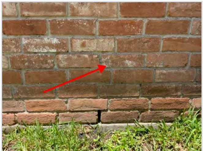
Brick crack (right side)
