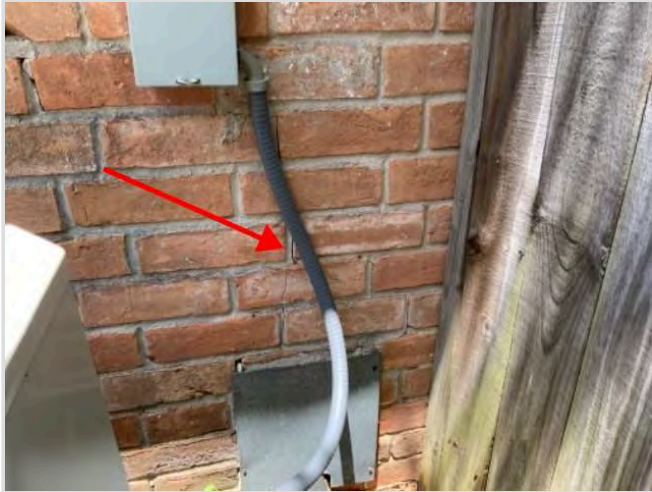
Brick crack (right side)
