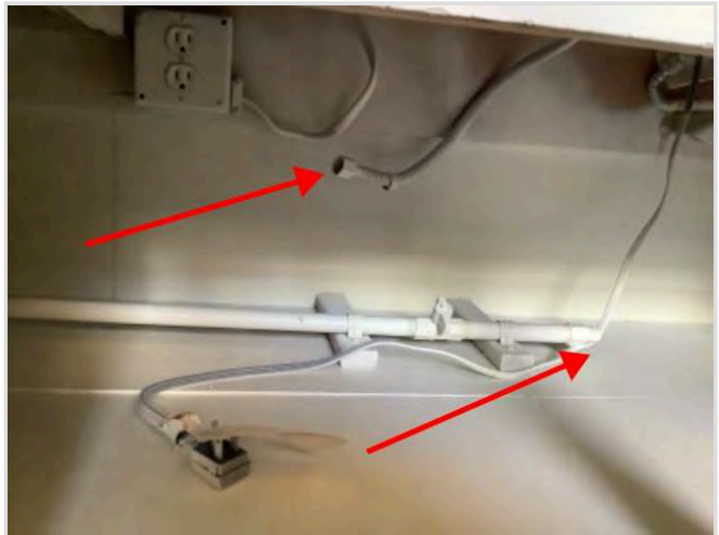
Gas line to cooktop was disconnected
