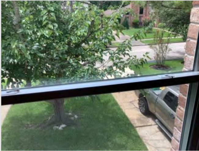
Window locks were non-functional (second floor front left bedroom)
