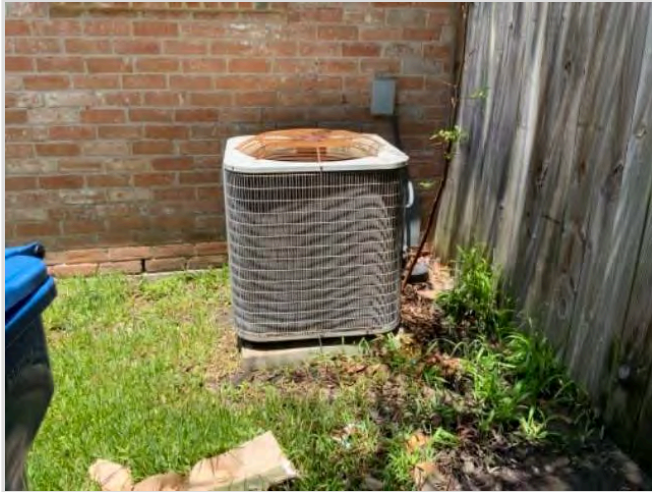
HVAC condenser unit (right side)
