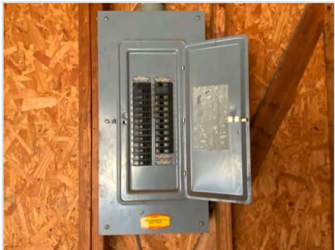
Electrical service panel
