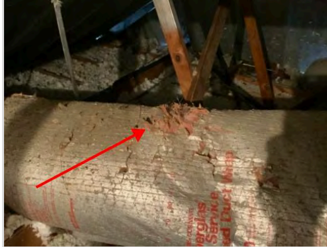
Damaged duct insulation
