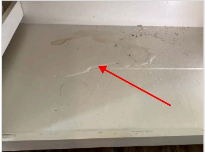
Leak (second floor bathroom sink)
