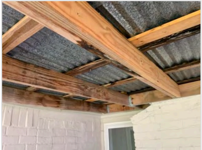
Signs of water penetration (back porch joists)
