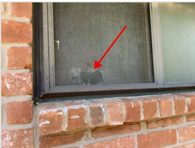
Damaged screen (right side)
