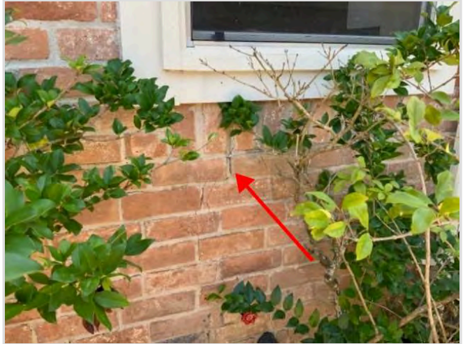
Brick crack (left side)
