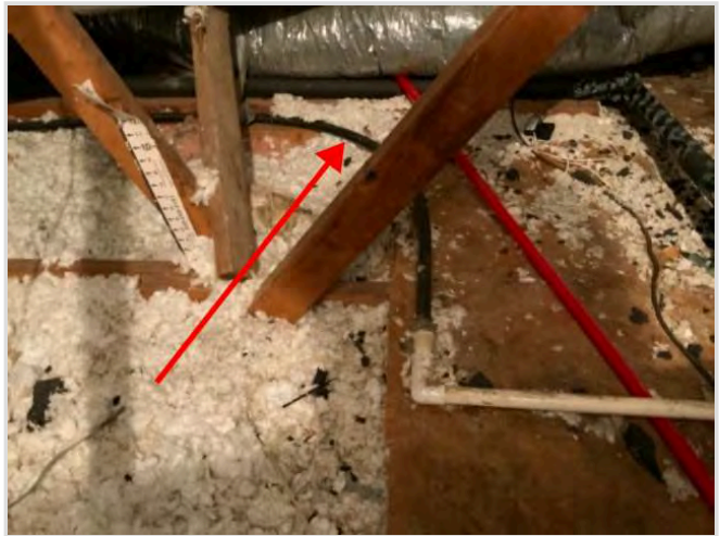
Flexible hose used for secondary drain line
