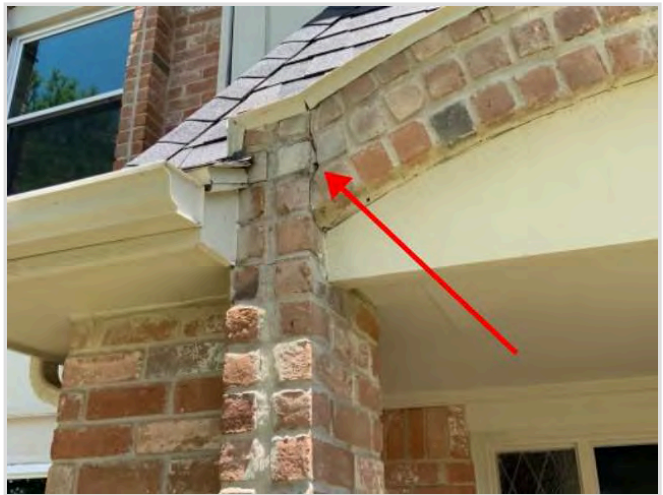
Brick cracks above front porch
