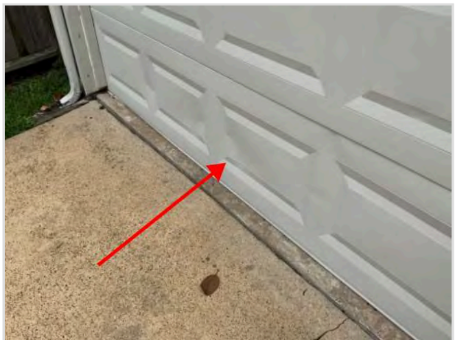
Damaged garage door
