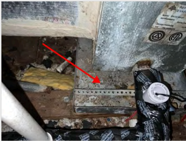
Secondary drain pan was showing signs of rust
