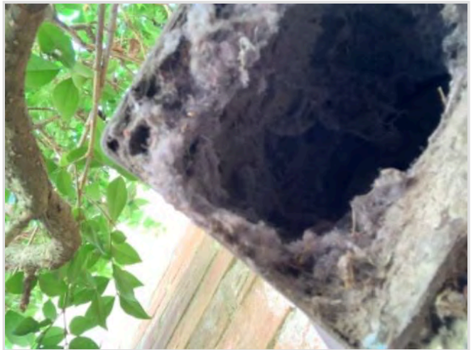
Dryer exhaust vent was missing damper and needed to be cleaned
