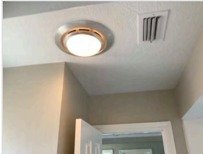
Exhaust fan was not working (second floor bathroom)
