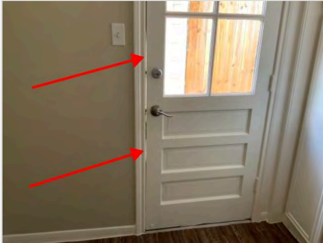
Missing weatherstripping (left back door)
