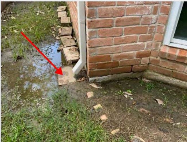
Missing splash pad (right side)
