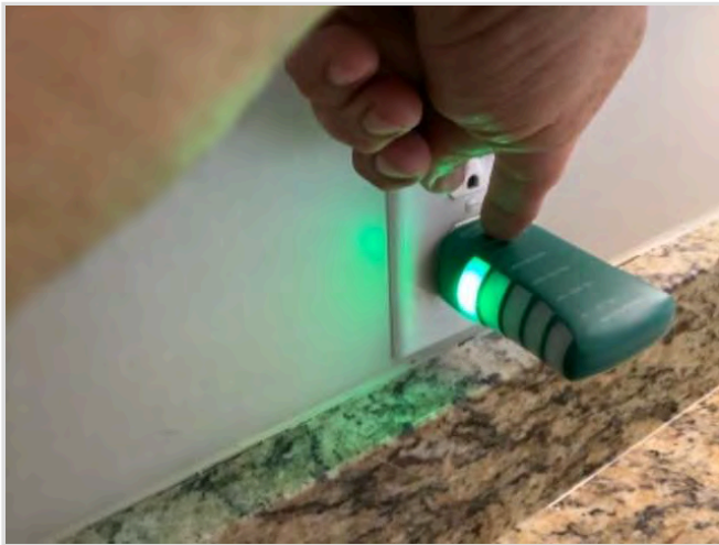
No GFCI protection (kitchen countertop)
