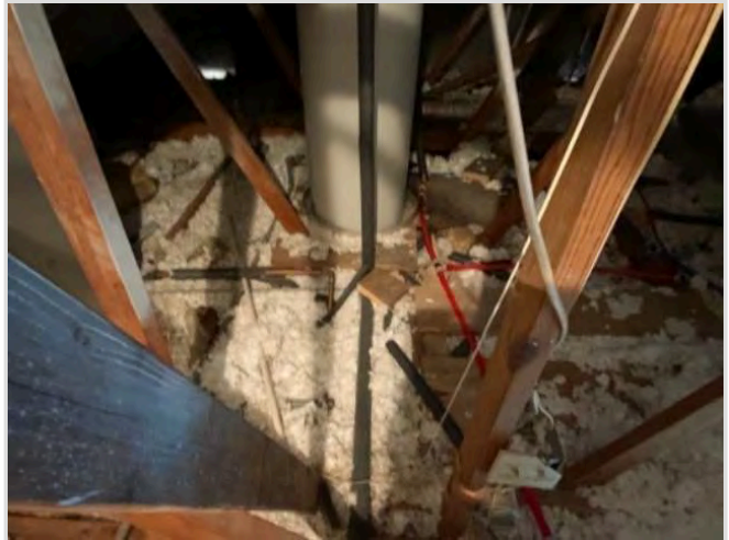
No floored passageway to water heater
