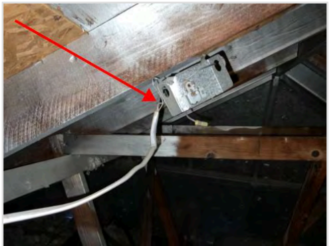
Wires outside of junction box (attic)
