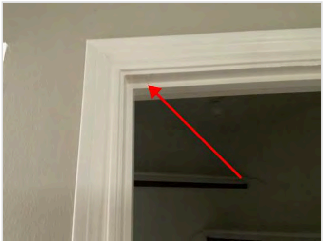
Door sticks / not square in jamb (master closet)
