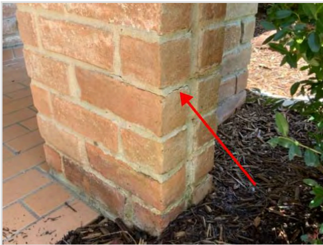
Brick cracks (front porch column)
