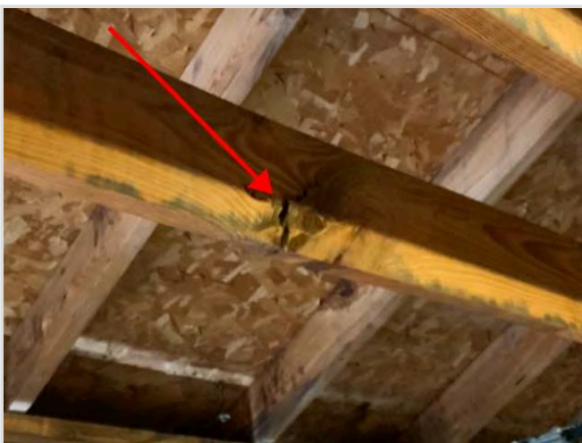
Damaged joist (garage)
