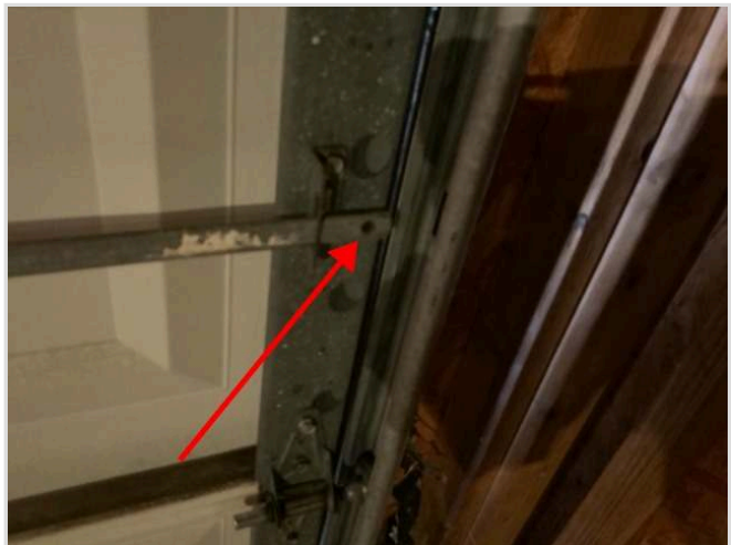
Garage door lock was not disabled
