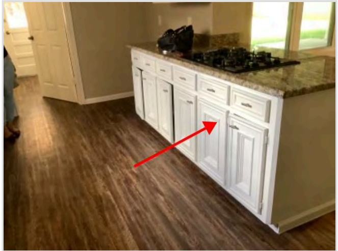
Cabinet door pull was missing (kitchen)
