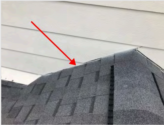
Siding in contact with roof covering (rear)
