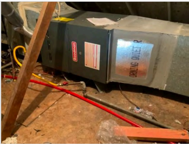
Furnace in attic
