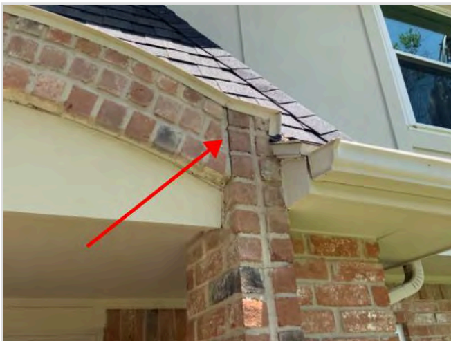
Brick cracks above front porch
