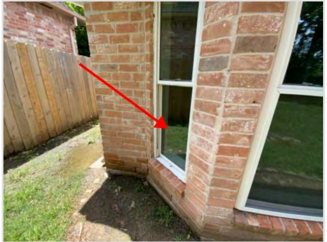
Missing screen (rear)
