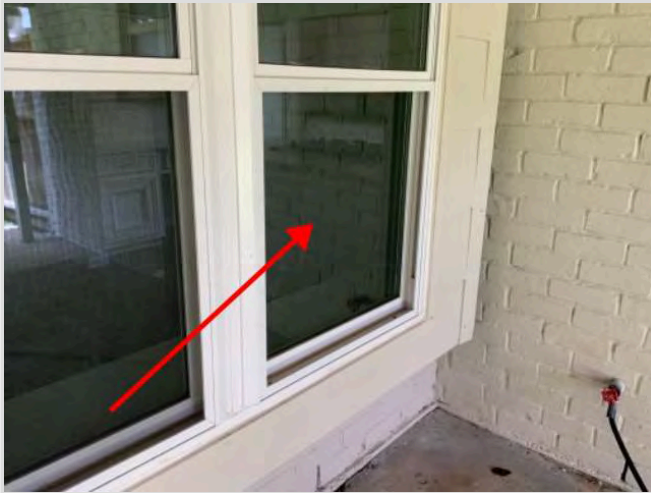
Missing screen (back porch)
