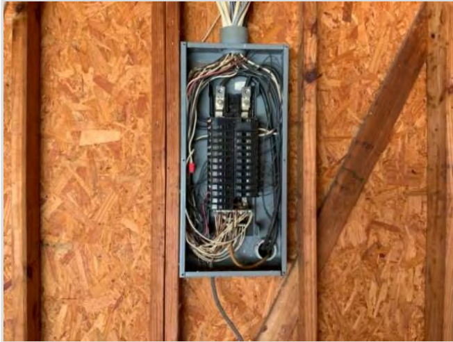
Dead front cover removed for inspection
