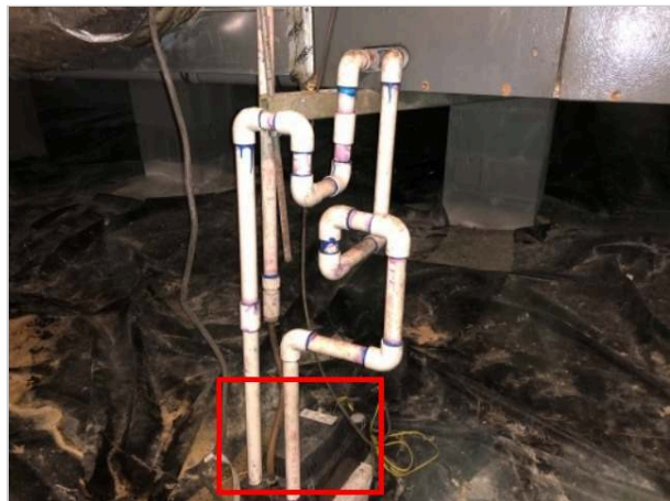
Pump at other system
