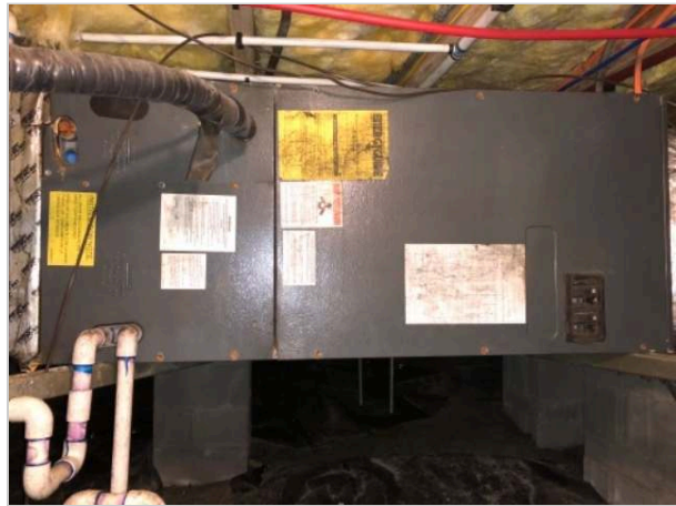
Left side indoor unit
