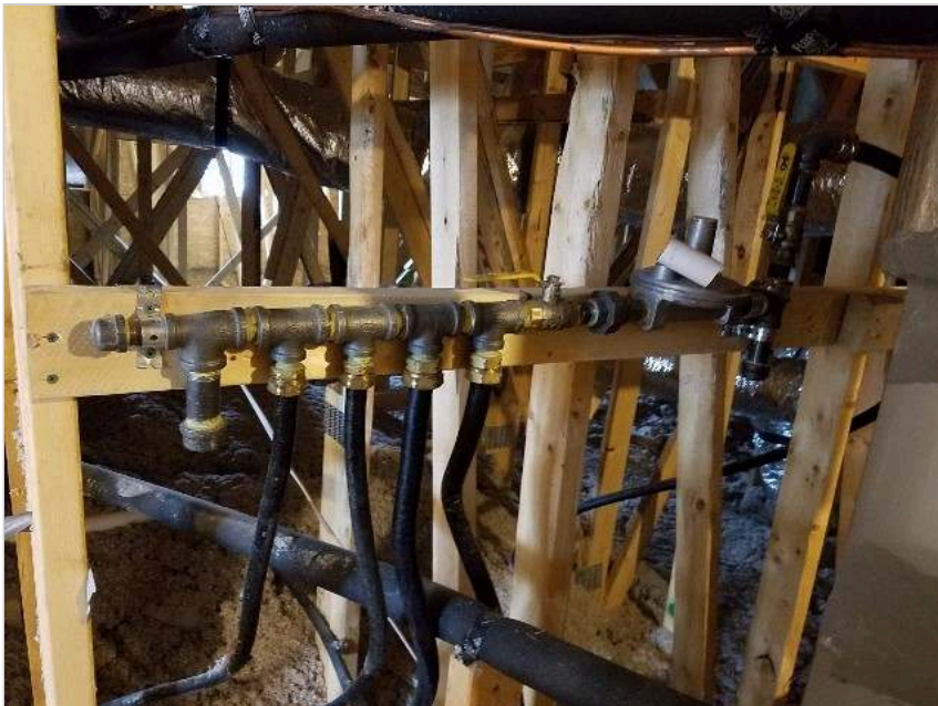
CSST manifold in attic space.
