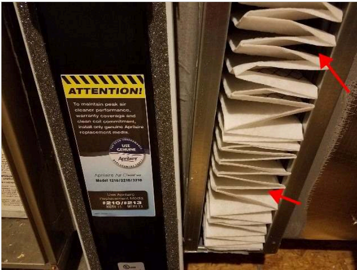
media filter installed backwards -- metal screen not facing suction side (upper HVAC unit).
