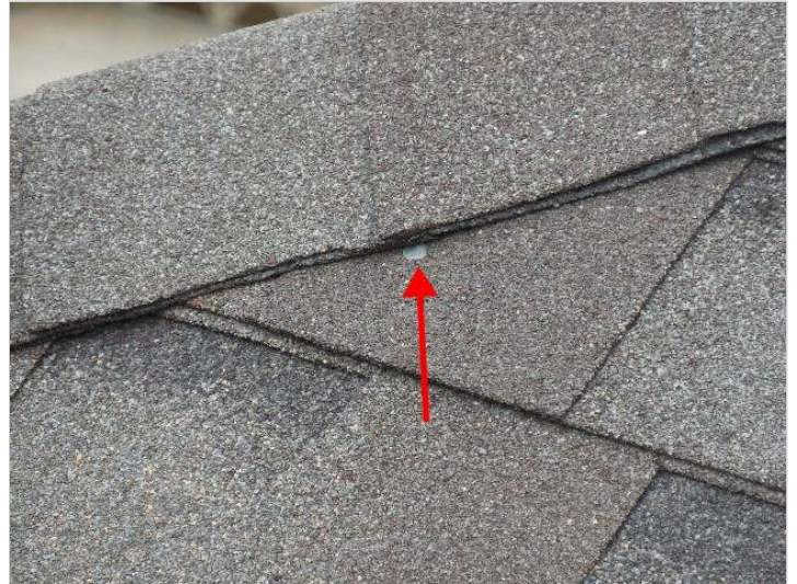
Exposed nail head on roof.
