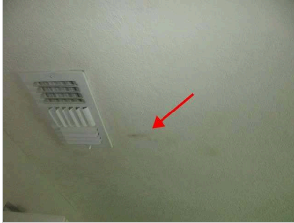
MOISTURE STAINS (DRY).
