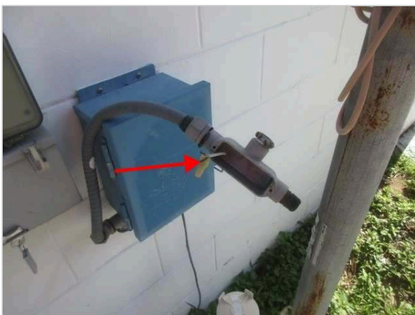
EXPOSED WIRES AT POOL EQUIPMENT
