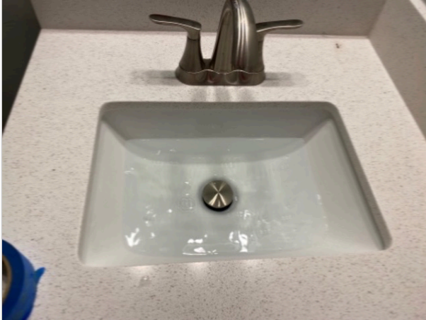
Hall bath sink drains slowly.
