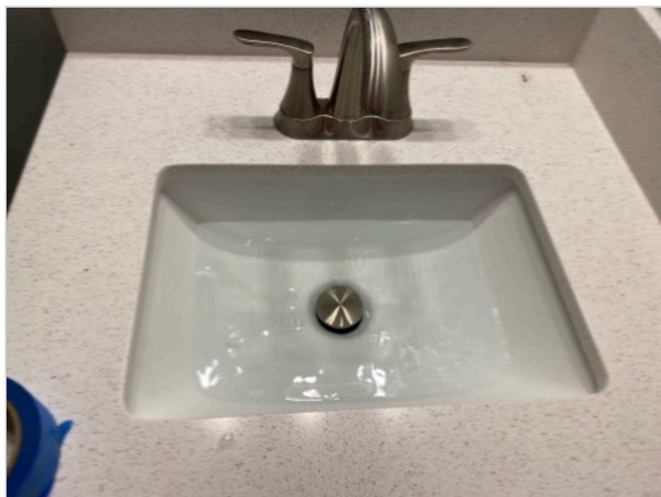
Hall bath sink drains slowly.
