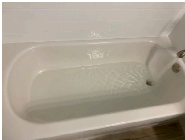
Hall bathroom drains slowly.
