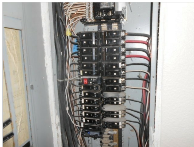
The electrical panel cover was removed for inspection of the house wiring, circuits and breakers.
