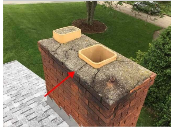
Mortar cap cracks - left chimney.
