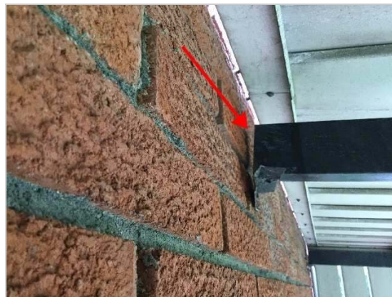
Awning supports not securely anchored to home.
