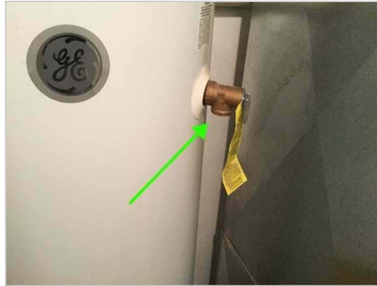
Missing drip leg.
