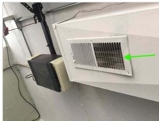
Open air ducts in garage.
