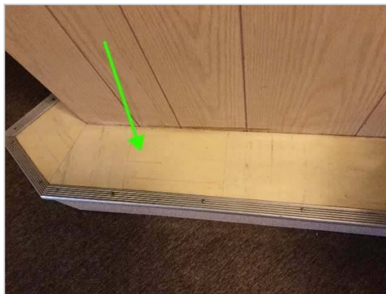
Possible asbestos tile.
