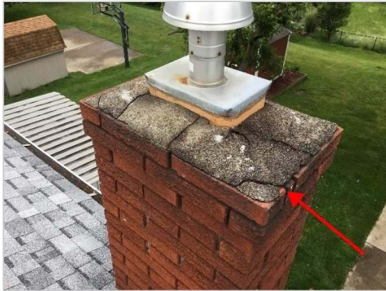
Mortar cap cracks - rear chimney.
