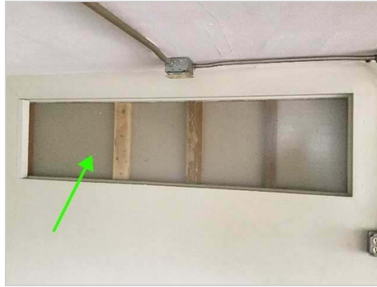
Non fire rated material in partition wall.
