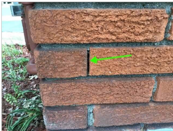
Missing mortar on home example.
