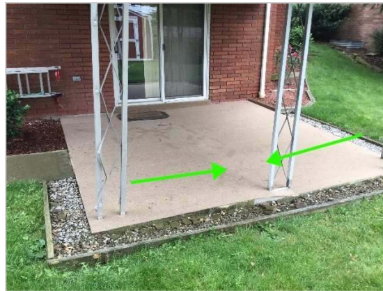
Patio slab settlement.
