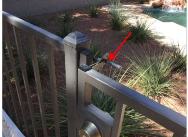
Gate Requires Adjustment
