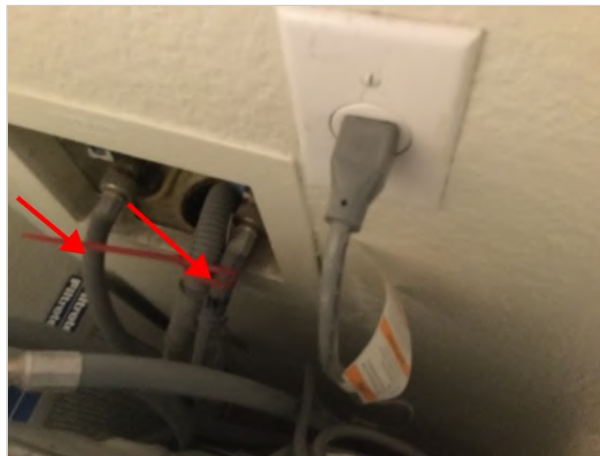
Washer Supply Hoses
