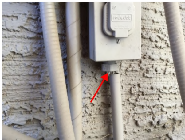
Pool Light Power
