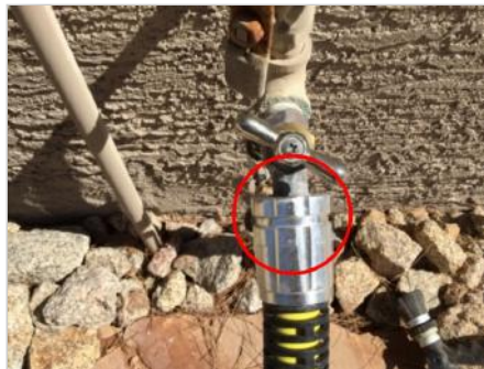
No Vacuum Breaker
