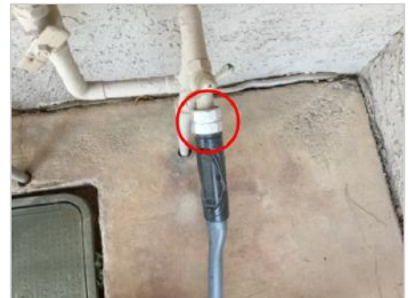
No Vacuum Breaker
