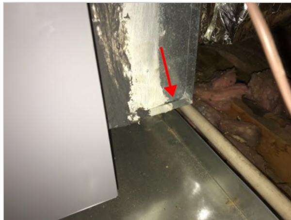
Right Side of Air Handler
