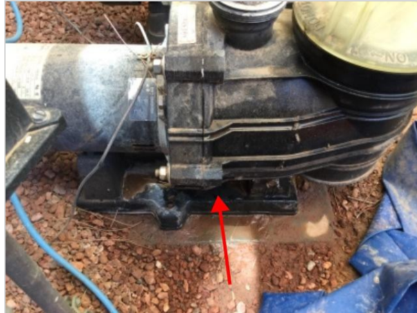
Water Feature Pump Leaking
