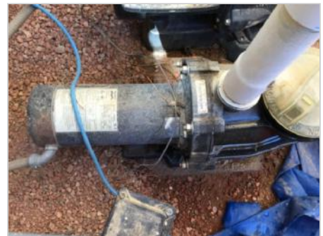
Water Feature Pump
