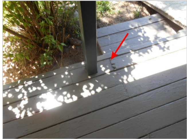
Loose or deteriorated deck boards on the rear deck.
