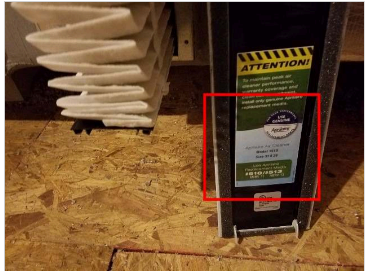
lower HVAC unit filter media type/size.
