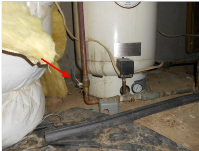
This is the main water shut off valve for the home.
