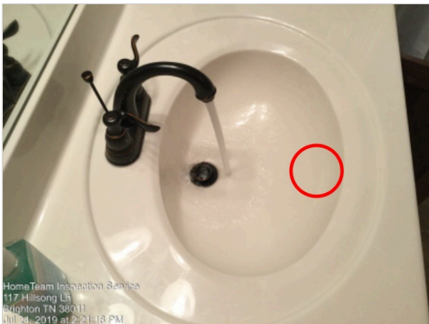
upstairs left sink
