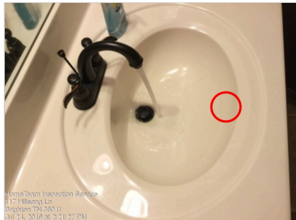
upstairs right sink
