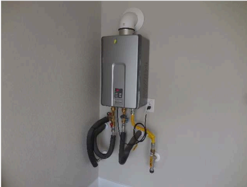
View of tankless water heater in garage.
