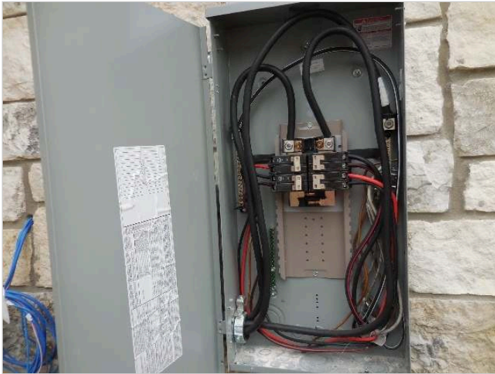
View of main electrical panel.
