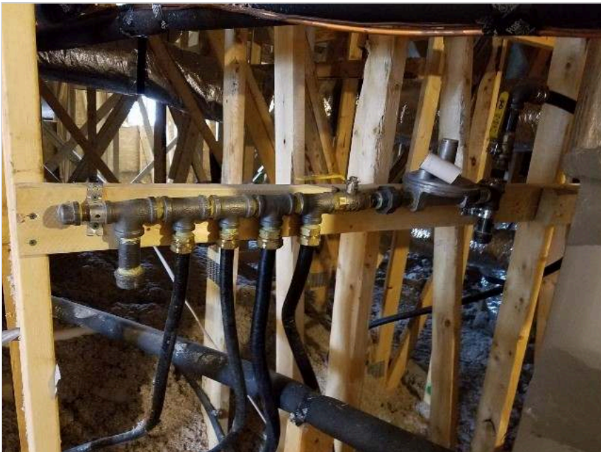
CSST manifold in attic space.
