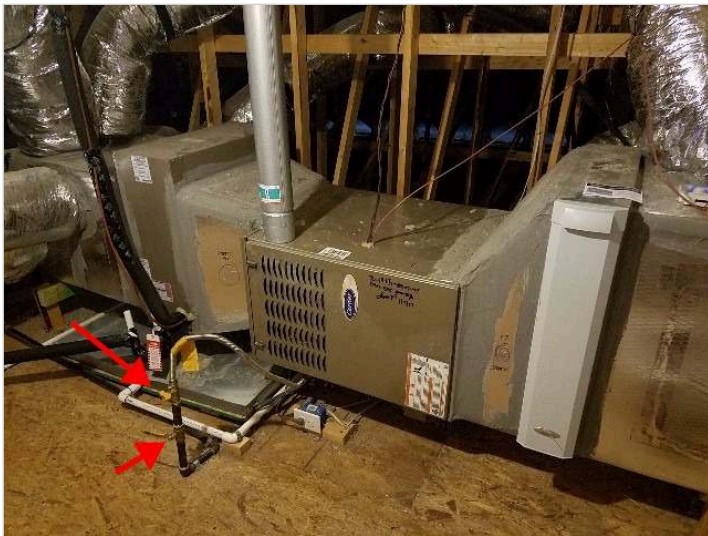
view of lower HVAC unit: gas and heater system off.
