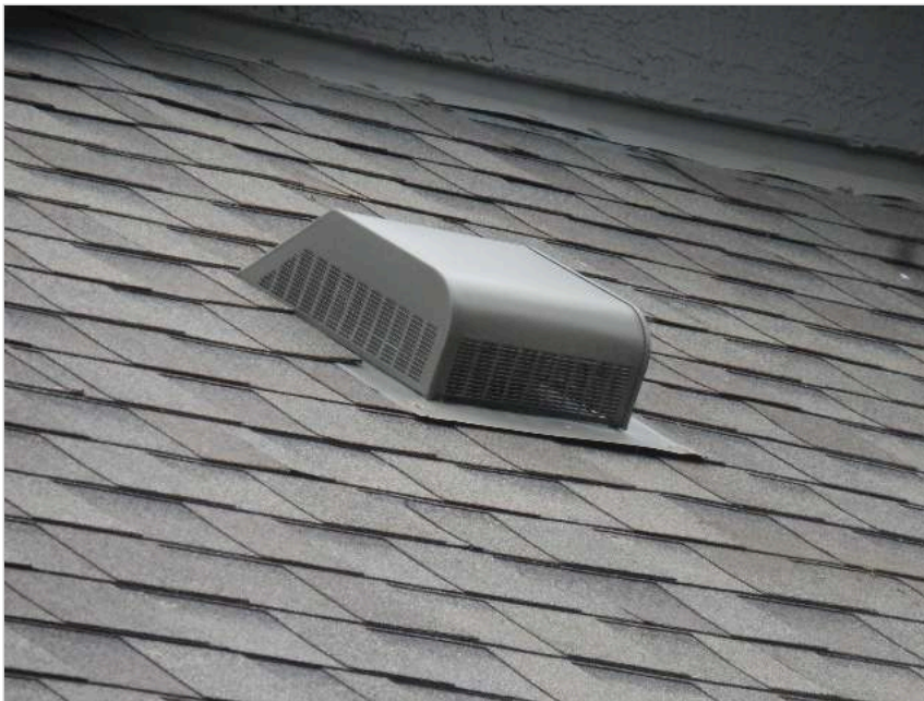
Screened dryer vent cover.
