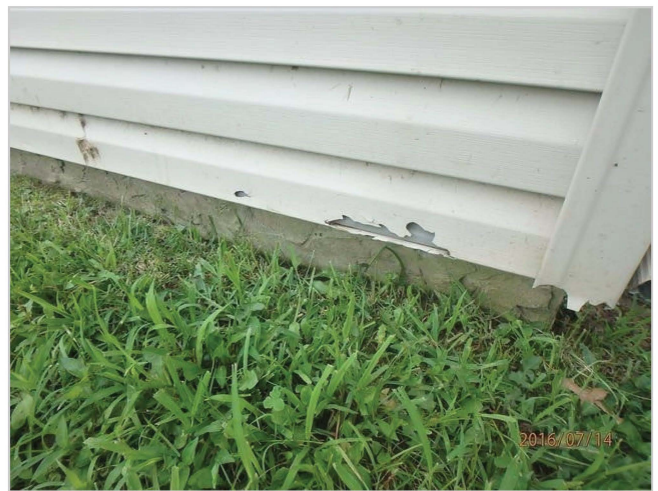
example of damaged siding
