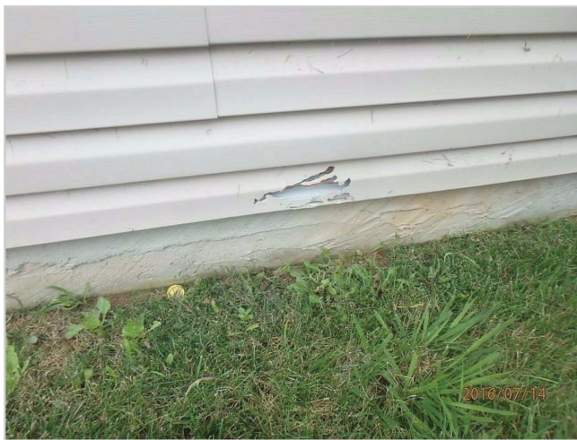
example of damaged siding
