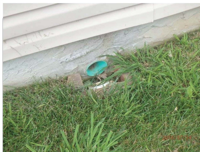
missing dryer vent cover
