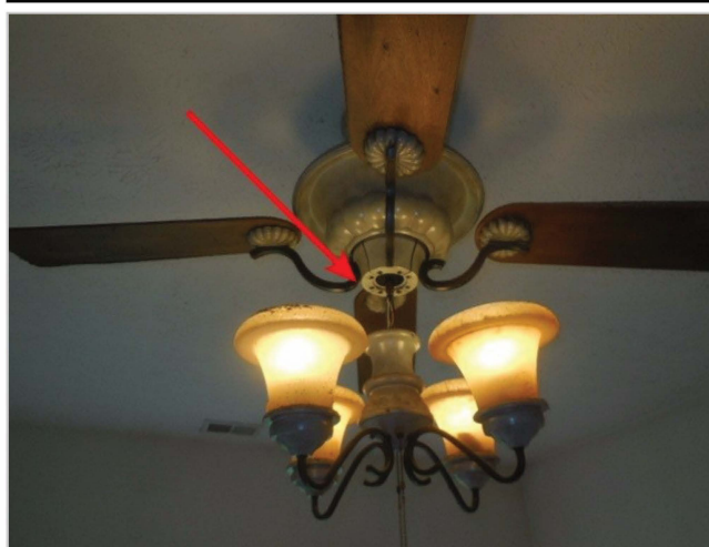
Loose light fixture.
