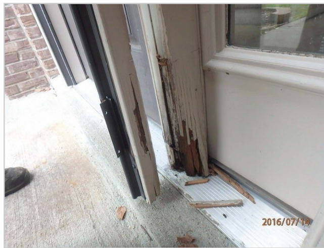
example of rotted wood around the front door
