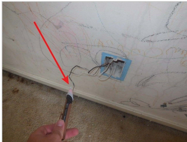
Exposed live wires.
