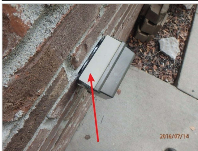
outlet is not properly covered
