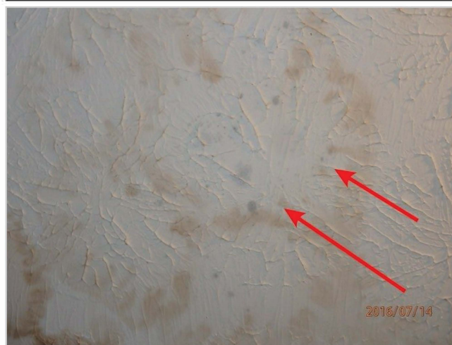
mold like growth in the garage
