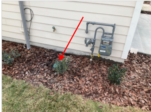
Water shut off
