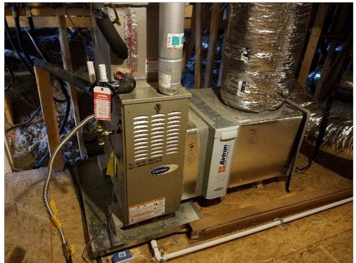
view of upper HVAC unit.
