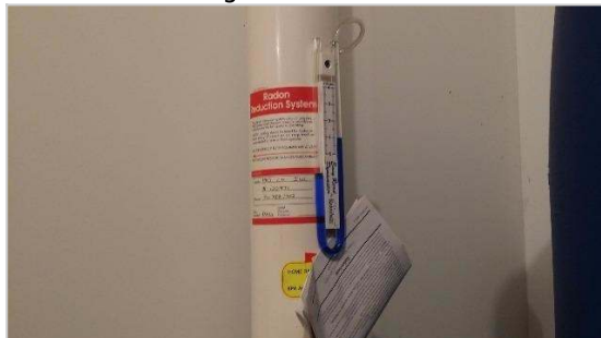
radon mitigation system monitoring station
