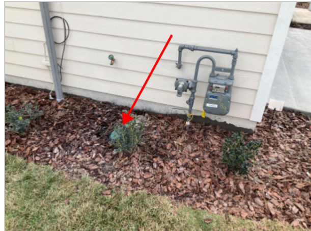
Water shut off
