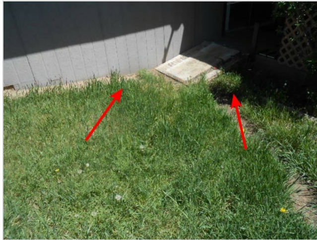
This area of exterior grading on the rear of the home is sloping towards the home.
