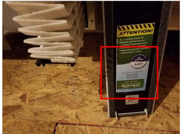
lower HVAC unit filter media type/size.
