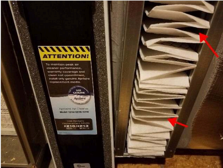
media filter installed backwards -- metal screen not facing suction side (upper HVAC unit).
