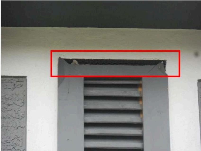
Part of trim damaged/missing at front gable vent.
