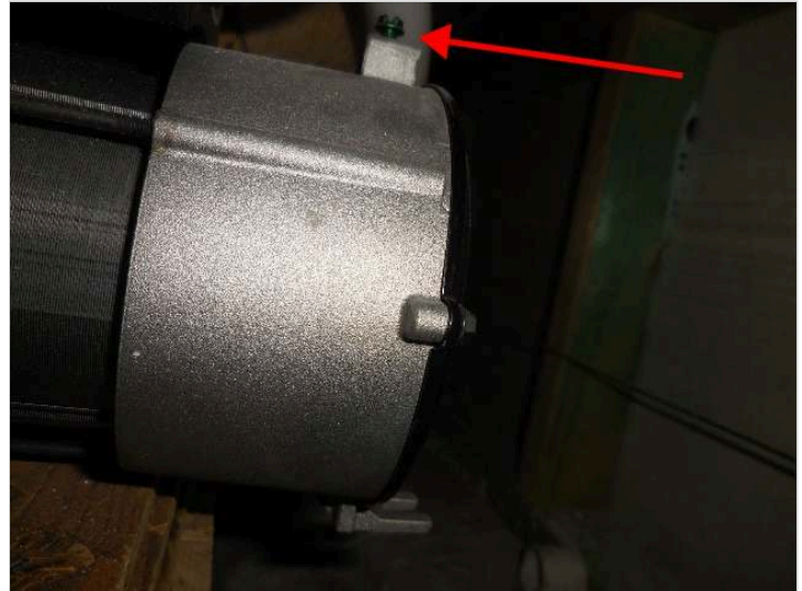
Spa tub motor not bonded.
