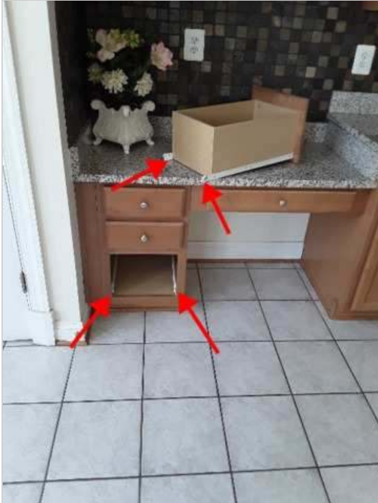
4. The latch was missing hardware on one of the door leading to the office on the main floor.
