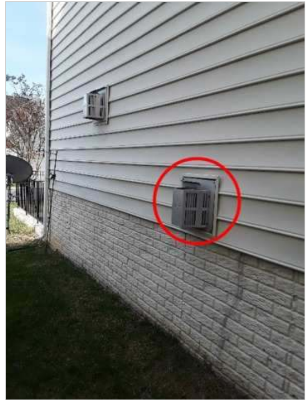
Direct vent for fireplace in basement
