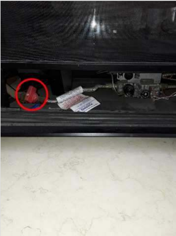
Main gas shutoff
