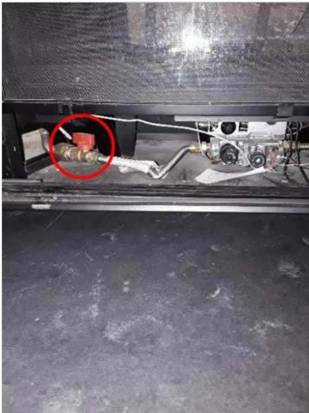
Main gas shutoff
