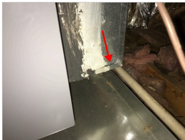
Right Side of Air Handler
