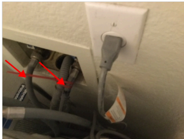
Washer Supply Hoses
