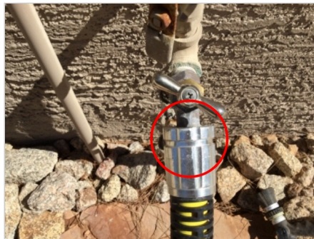
No Vacuum Breaker
