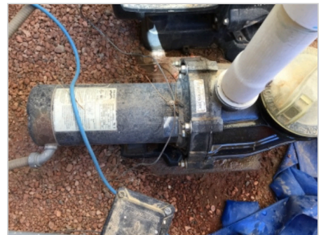
Water Feature Pump
