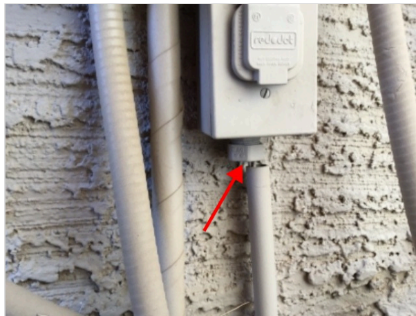
Pool Light Power
