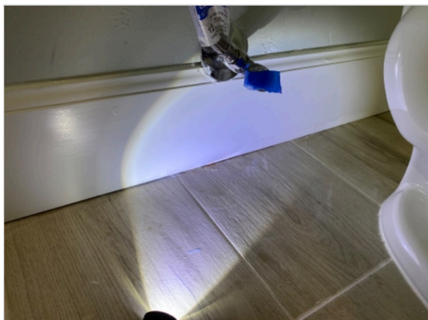
The Jack and Jill toilet shut off is leaking.
