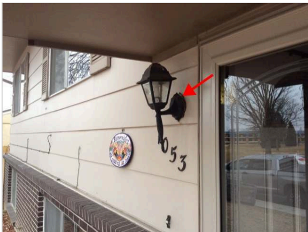
The front, exterior light fixture is loose from the wall.
