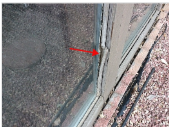
Deteriorated window frame.
