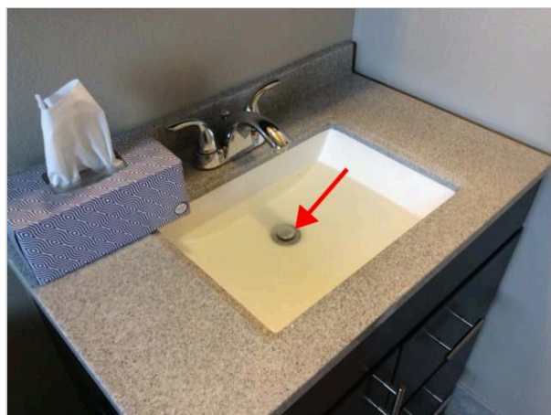
Sink drains slowly.
