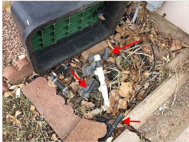
Disconnected lawn sprinklers and piping.
