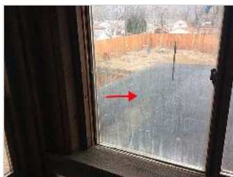
Broken window in the patio addition.
