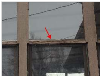
Deteriorated window frame.
