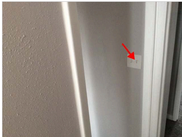
Three way switch for entry way light fixture is wired incorrectly.
