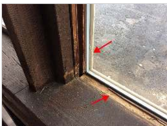
Deteriorated window guide and broken window in the patio addition.
