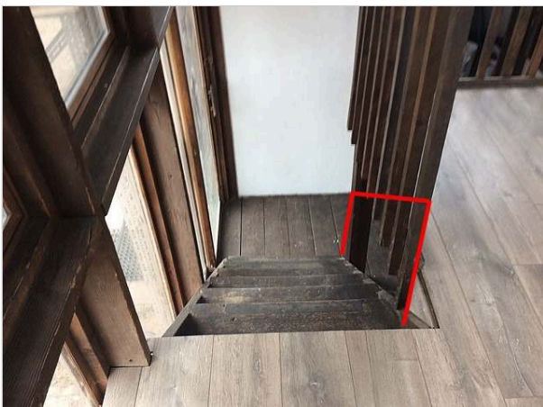
A safety railing would be recommended for this stairway in the patio conversion.
