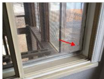
Hole in the window in the kitchen.
