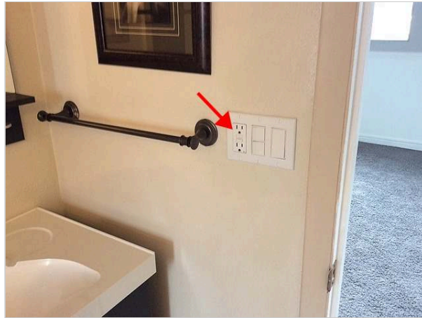
Non functional GFCI receptacle.
