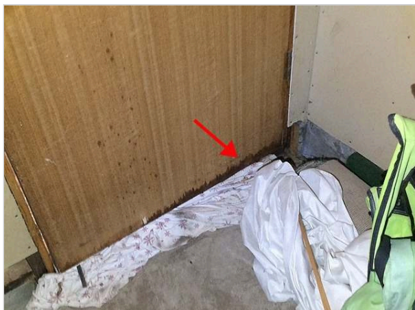
The rear garage exit door is water damaged along the bottom.
