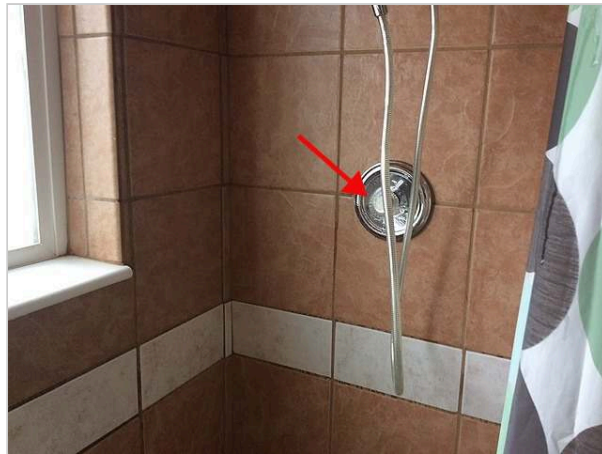
Shower valve is out of adjustment.
