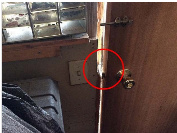
And the door does not close, latch or lock.
