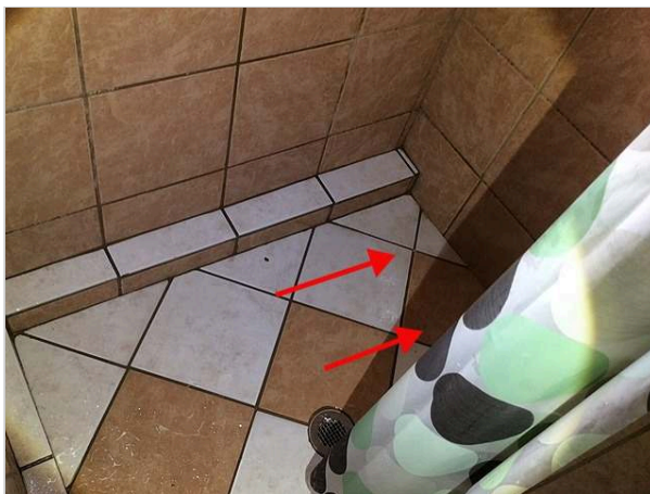
The shower pan slopes towards the wall instead of the drain.
