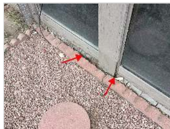
Deteriorated window frame.
