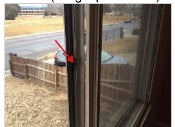
Missing lock on bedroom window.
