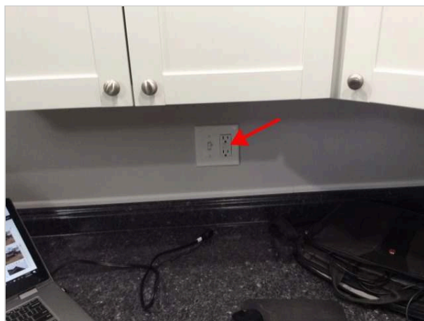
Electrical receptacle does not have power.
