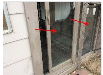
Broken glass on both glass doors ( single pane now )
