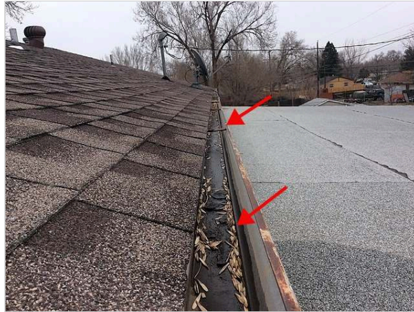
Rusted gutters were common throughout.
