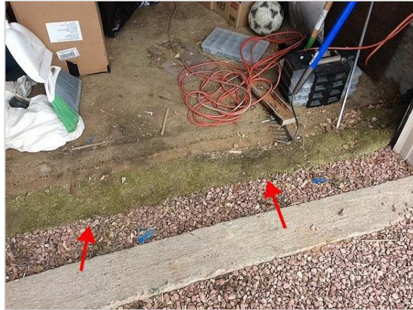
The garage floor is only constructed of carpeting over rock.
