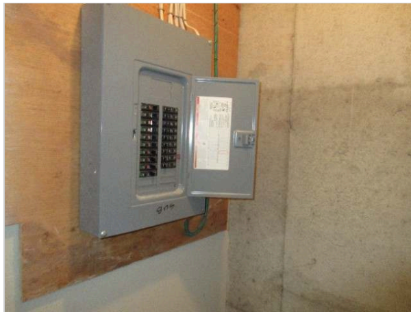
basement sub panel
