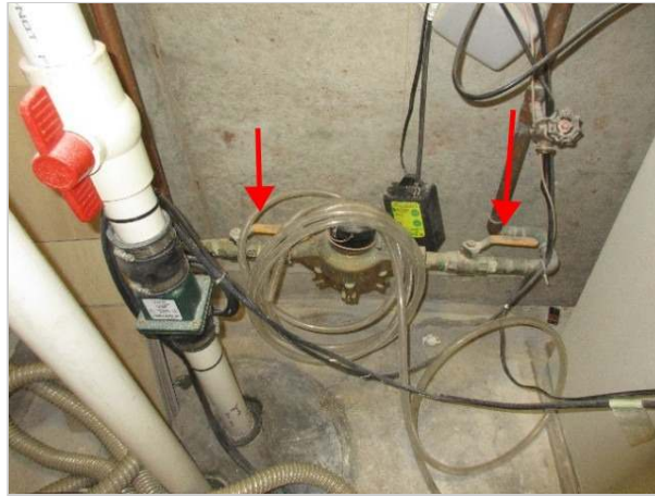
water shutoff valves
