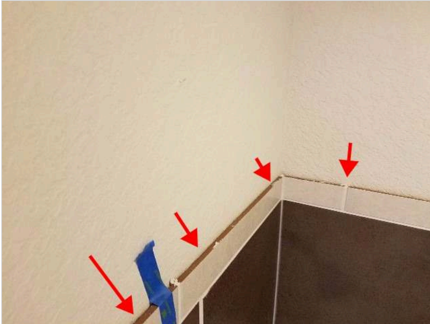
example of unsealed/caulked gaps at top of shower enclosures.
