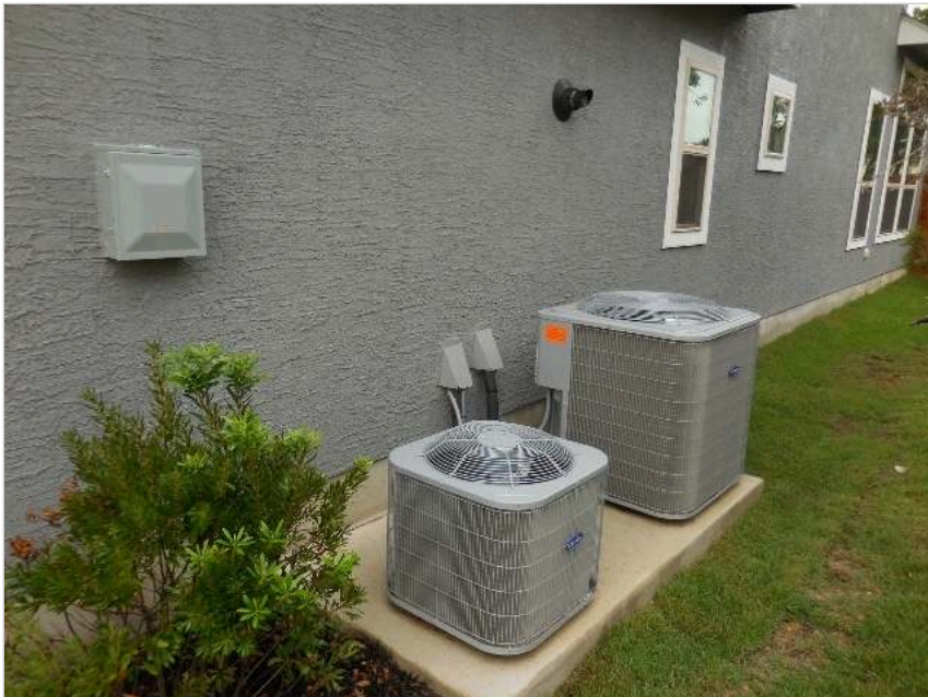
View of condenser units.
