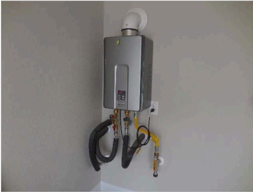
View of tankless water heater in garage.
