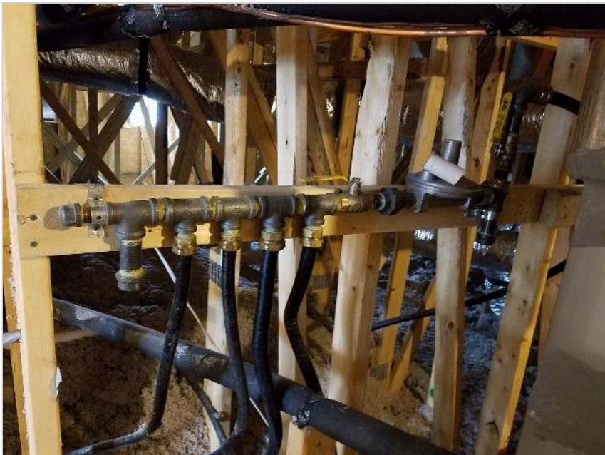
CSST manifold in attic space.
