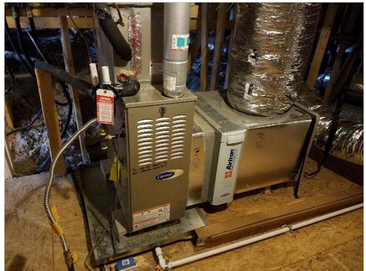
view of upper HVAC unit.
