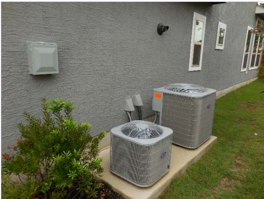
View of condenser units.
