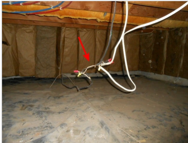
Open spliced wiring in the crawlspace.
